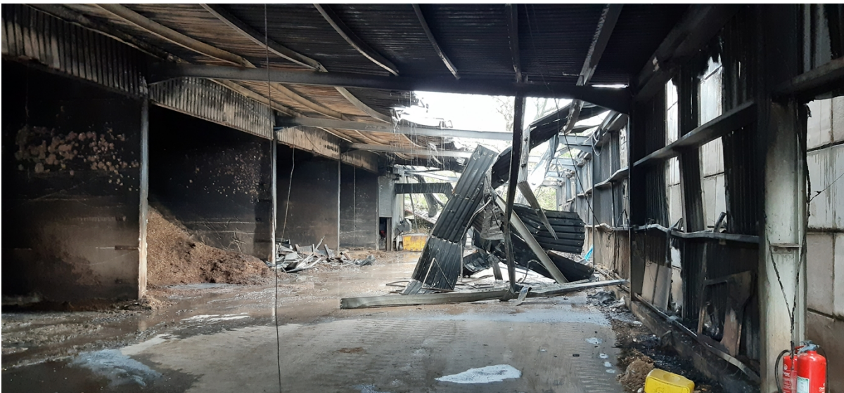
Photo 5 - Photo of fire incident taken by NRW Officer Greg GARDNER on 01/11/22
