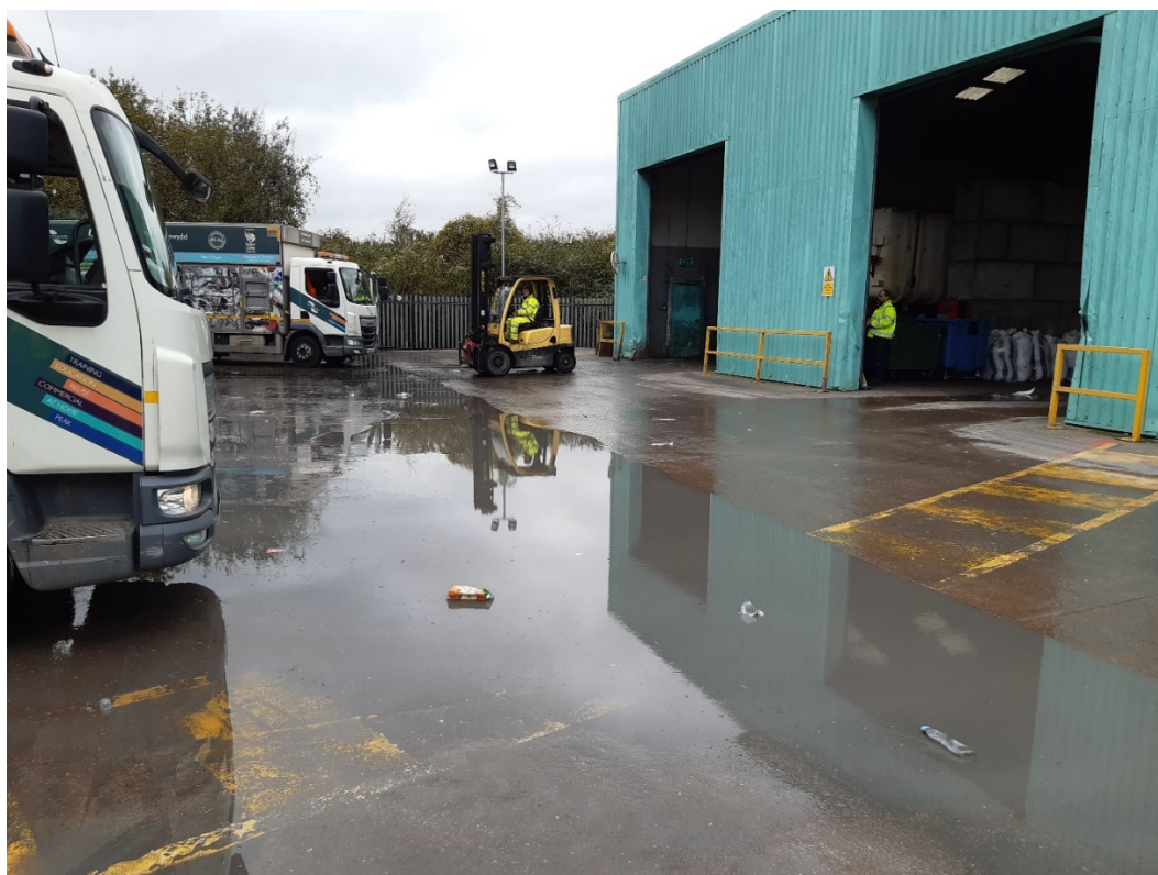
Photo 2 – standing water in the yard due to blocked drainage channels
