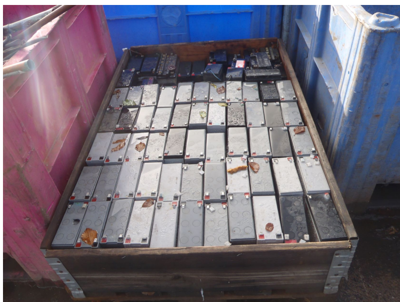
Battery storage box
