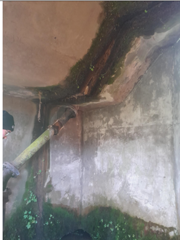
Image of the effluent leak under the asset.
