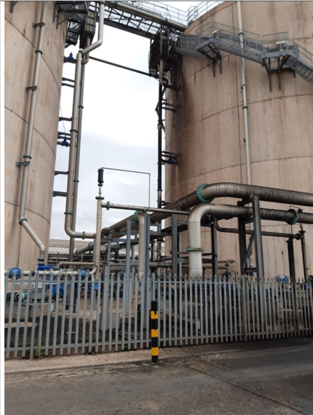
Picture 3: Image showing the weir box overflowing. Image also shows the extent of the digestate falling down the side of the digester and on the roads on site.
