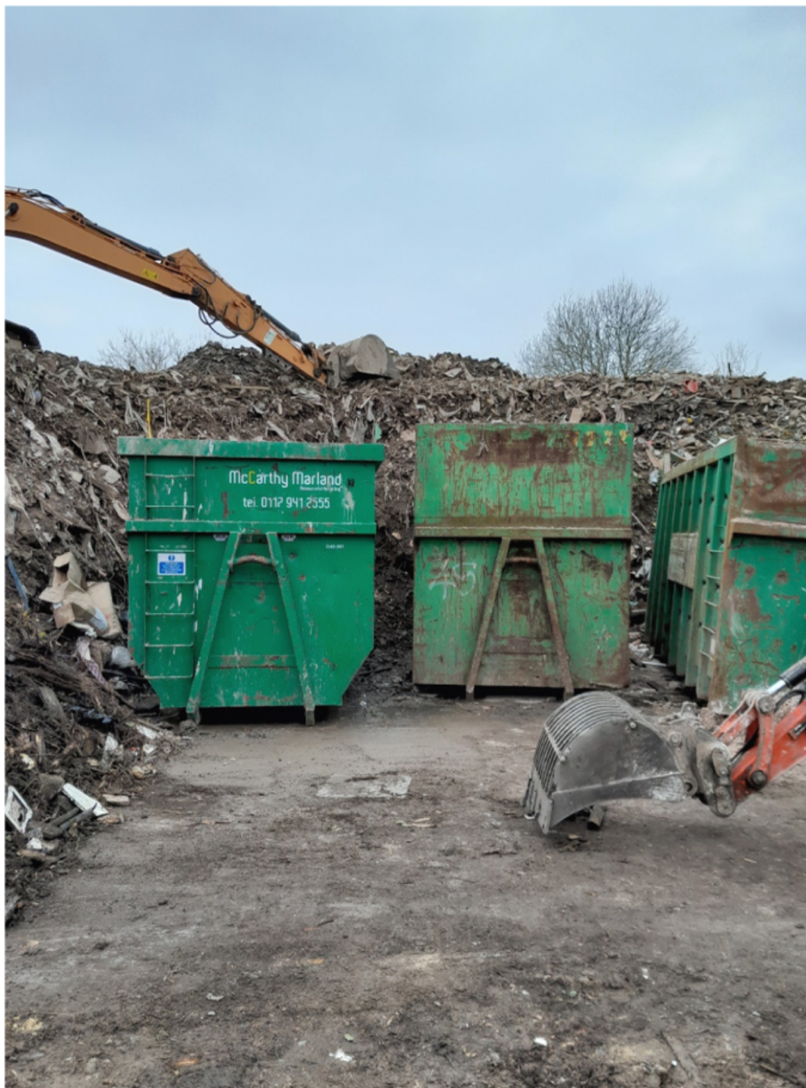
Images 1,2 & 3 showing the height of the waste pile (Image 1)
