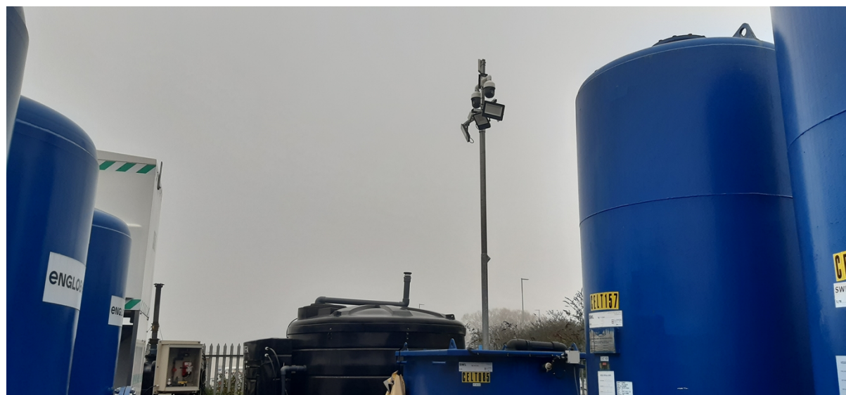
Photo 3 - Security cameras with 360-degree vision and floodlighting
