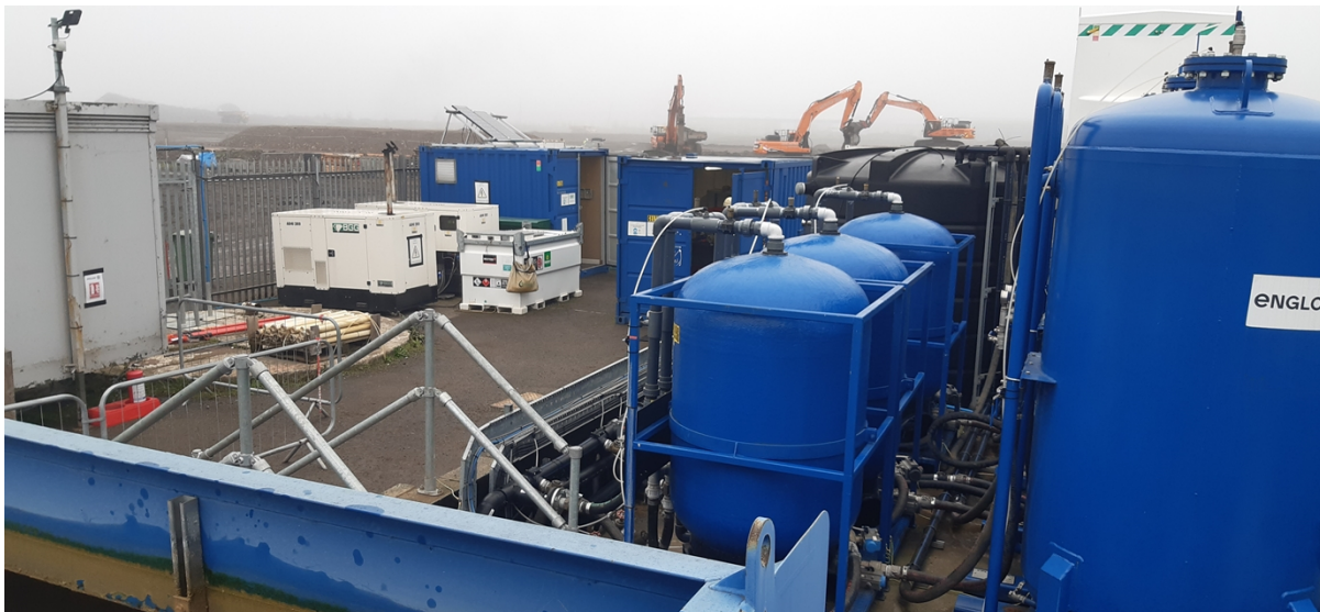
Photo 1 - Englobe filter tanks for contaminated water
