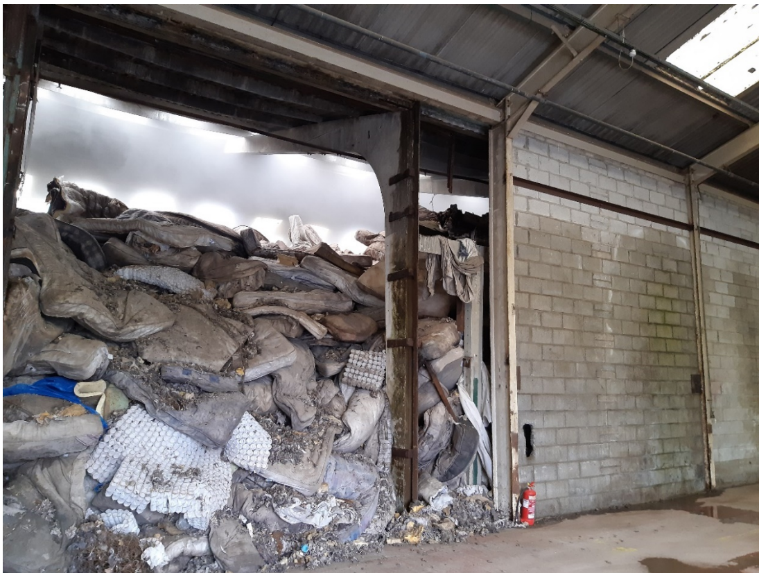
Photo 3 - Behind the brick wall is the storage of RDF next to the mattresses and the resulting heat from the RDF waste.
