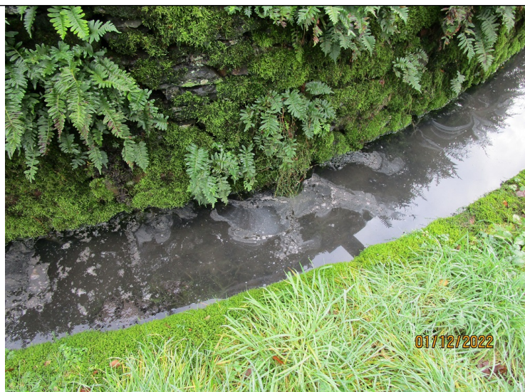
Photo of stagnant final effluent 'moat' around filter beds.
