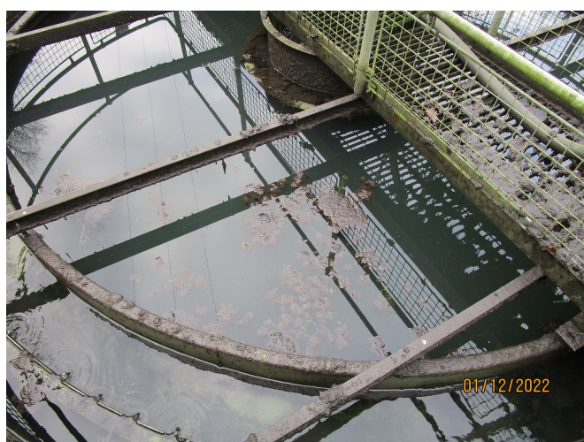
Photo of condition of final effluent tank, with clear signs of mud deposit in and around tank, from fluvial flooding.
