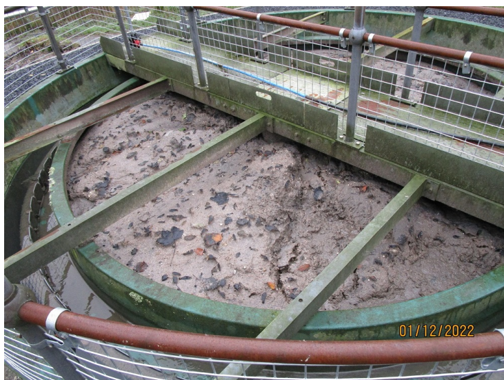
Photo of primary tanks with excessive volume of sludge.
