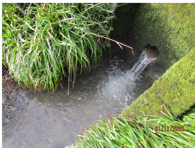
Photo of final effluent outfall
