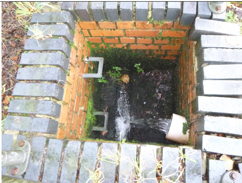
Photograph 6: Final effluent sampling point
