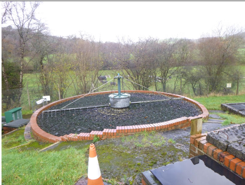
Photograph 4: Stone media filter bed 2
