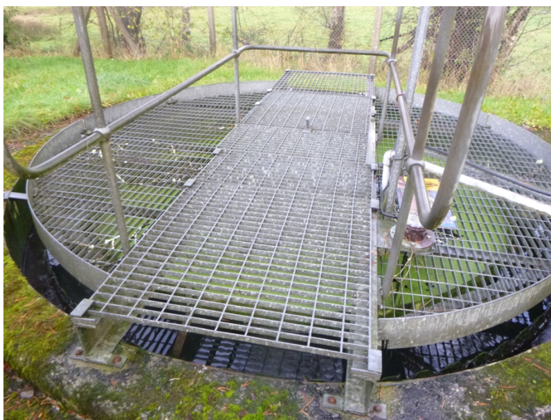
Photograph 5: Final settlement tank (FST)
