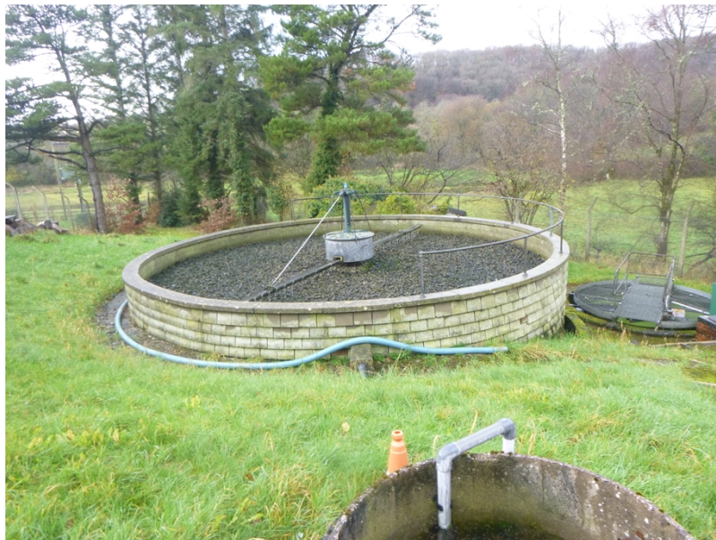
Photograph 3: Stone media filter bed 1
