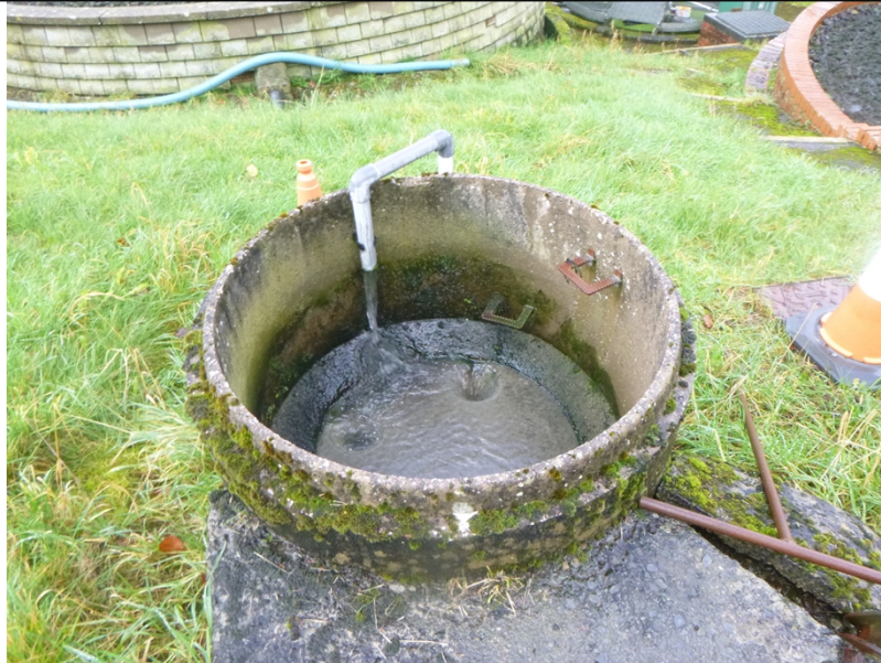
Photograph 2: Distribution chamber supplying two filter beds (seen in the background)
