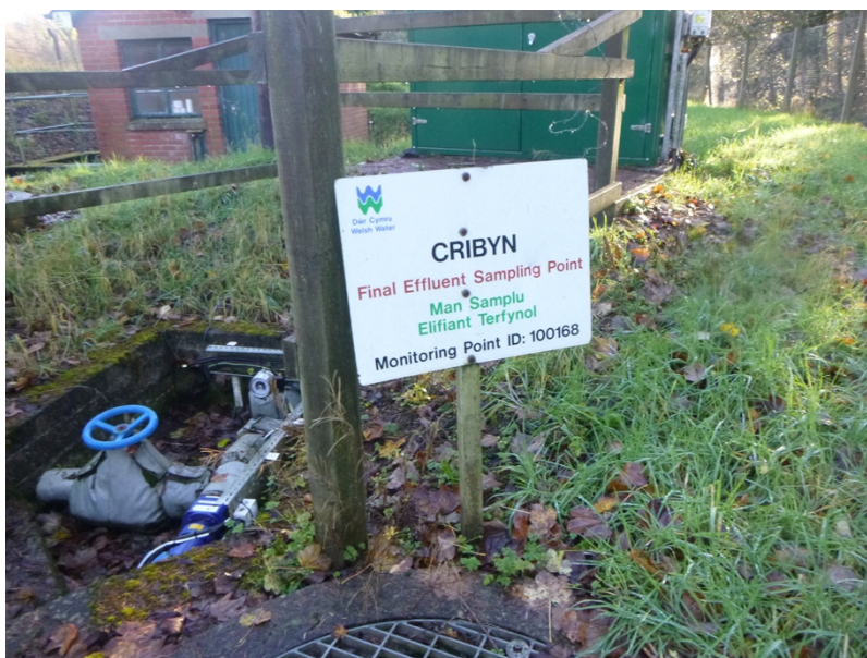
Photograph 7: Final effluent sampling point
