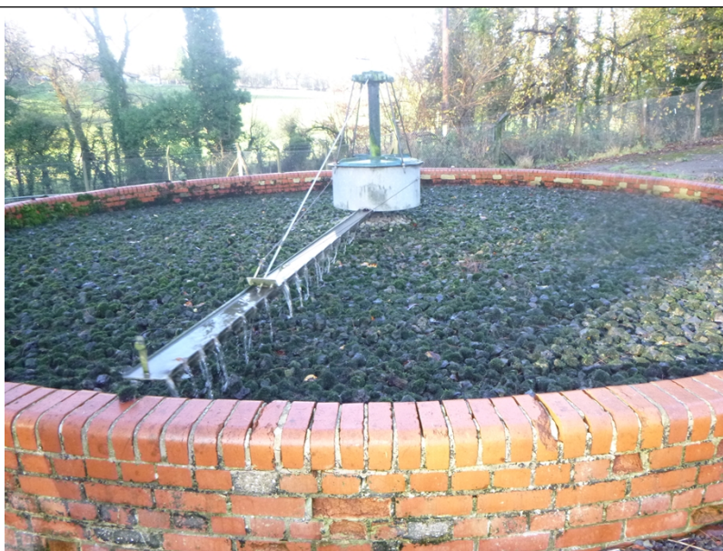
Photograph 4: Stone media filter bed
