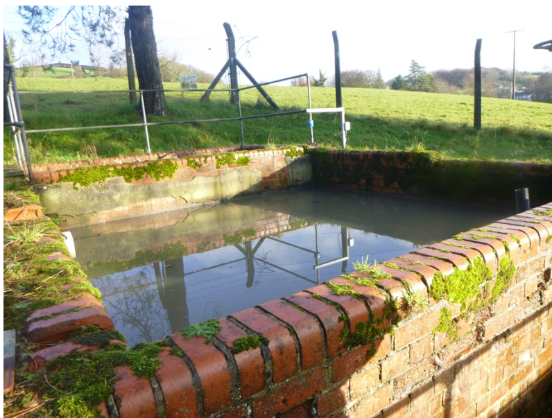
Photograph 3: Sludge holding tank
