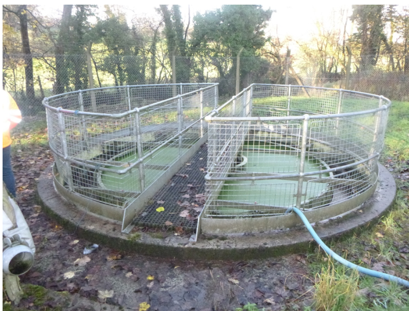
Photograph 5: Final Settlement Tank (FST)
