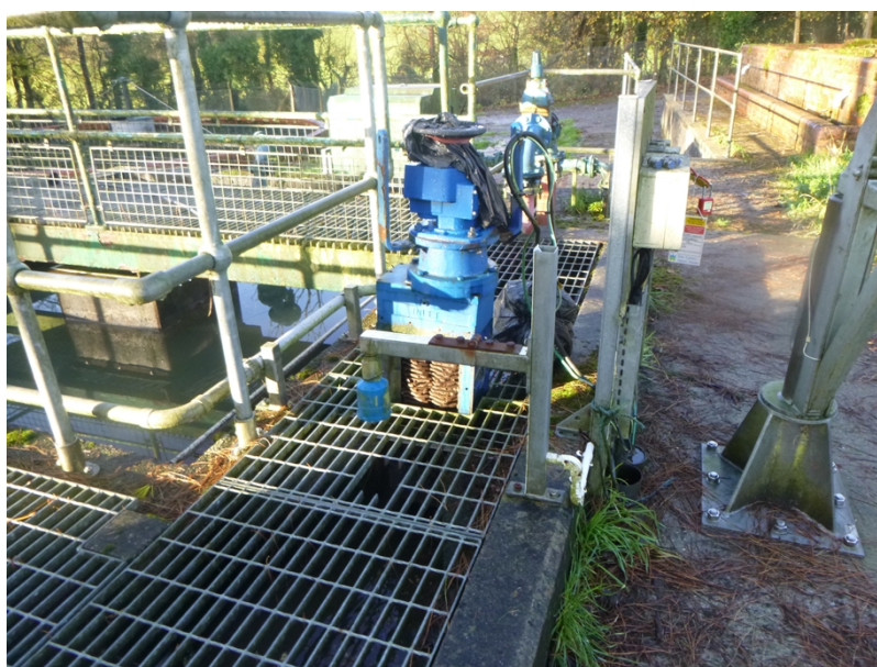
Photograph 1: Muncher (blue) and Primary Settlement Tank (PST)
