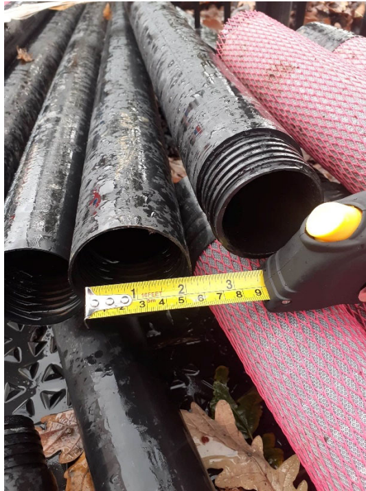
Photograph 5 63mm outer diameter 51mm internal diameter plain HDPE pipe
