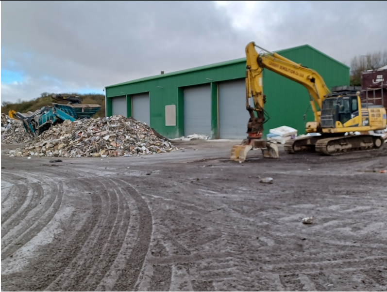
Photo's above showing infrastructure and leachate
