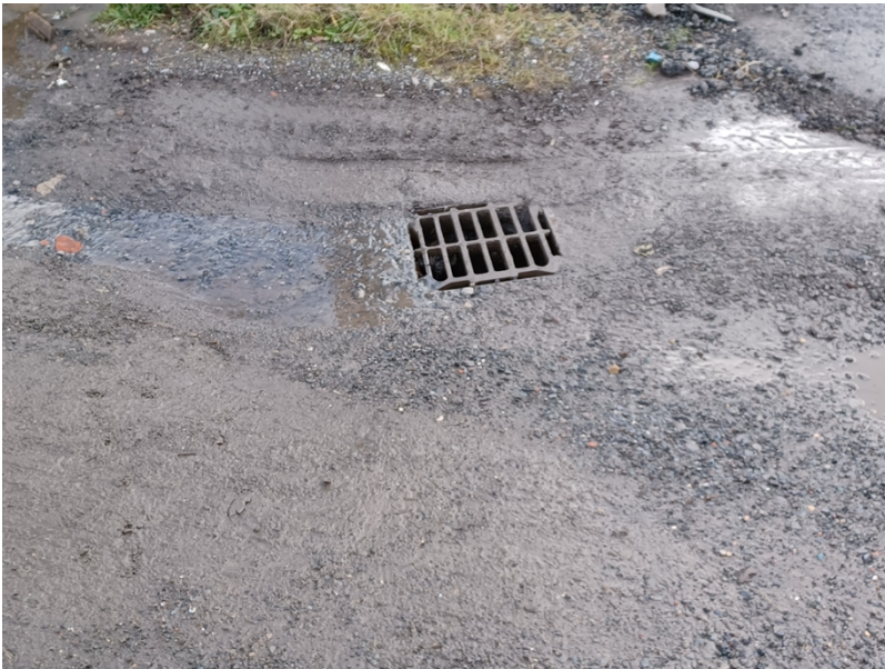
Photo above taken on hardstanding area showing run off entering drain and by passing off site
