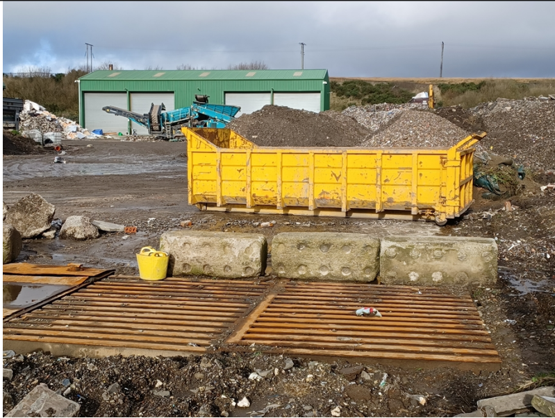
Photo above showing drainage with unmade ground around it, run off able to by pass.
