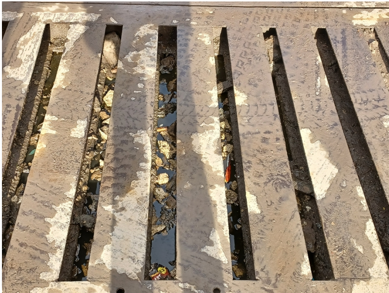
Photo above showing silt trap and interceptor blocked
