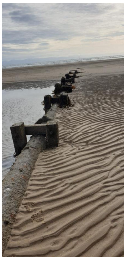
Figure 2 – Outfall pipe - The damaged pipe is 100m from this point towards the marker seen out at sea (end of the sewer pipe).
