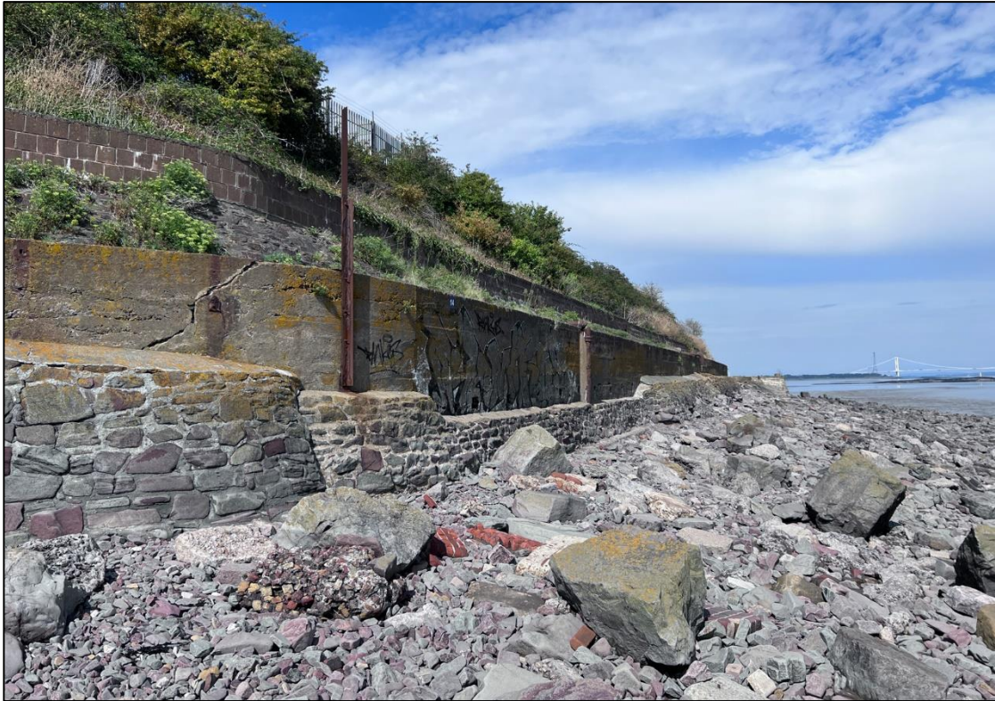
Figure 6: Down stream tiered defence wall and some rock armour (rock armour appears to have been displaced)
