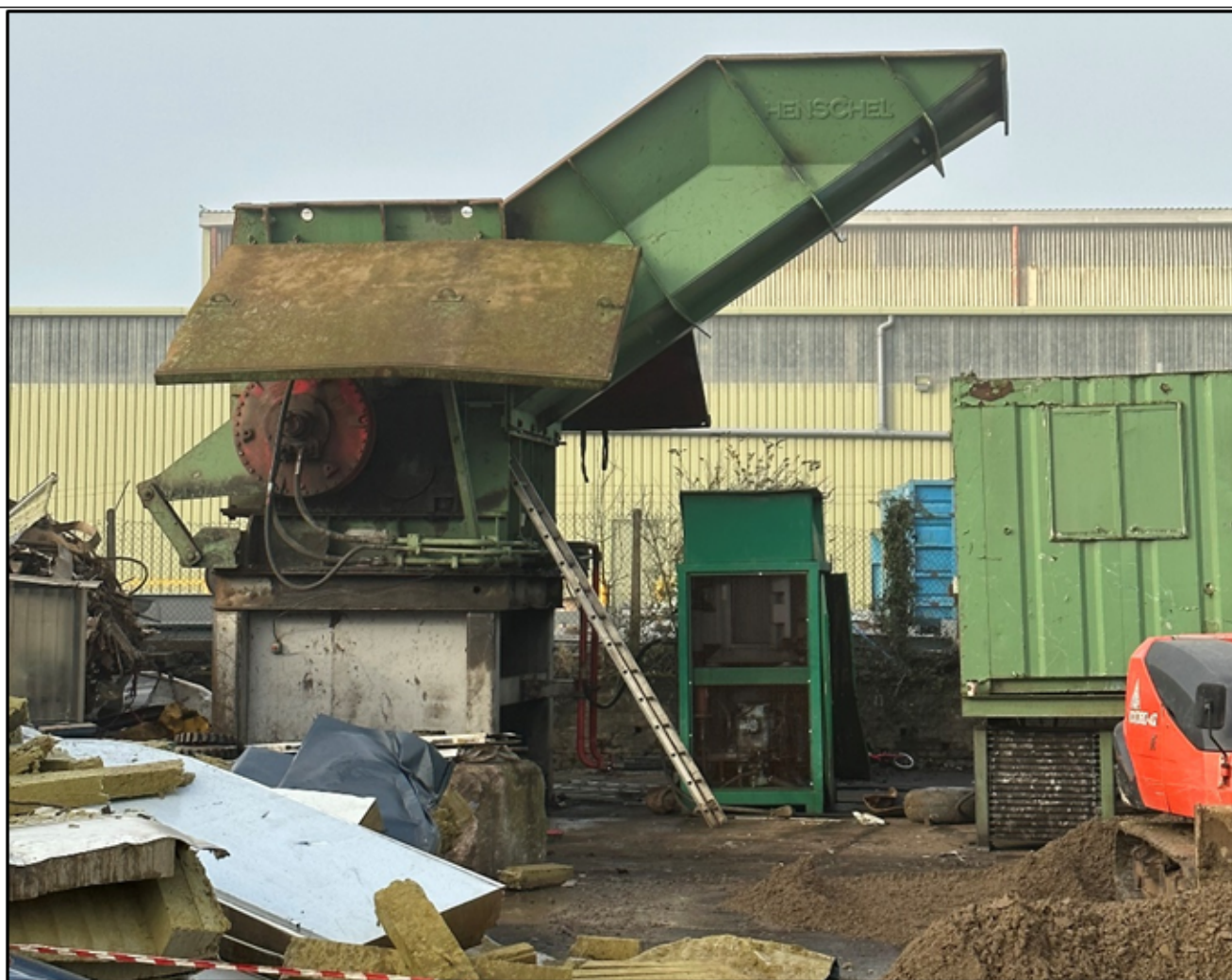
Image 3 – showing pre-shredder equipment installed and in-use on site
