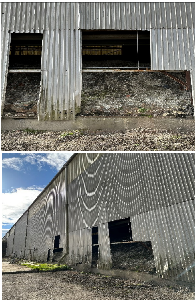
Images 1 and 2 - showing building unit missing panels with waste exposed and accessible
