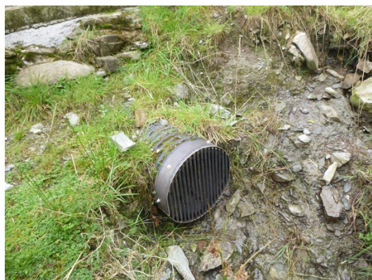
Figure 3: Discharge outlet pipe and new screen
