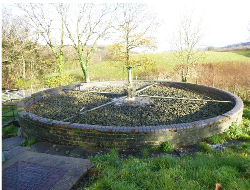
Photograph 2: Stone media filter bed (prior to arm clearing)
