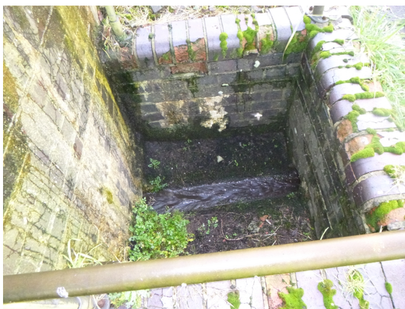
Photograph 4: Final effluent discharging from the filter bed
