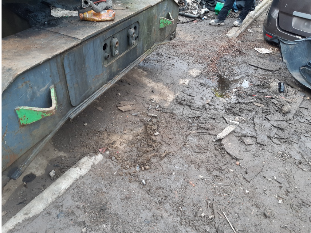
Photo 1 – damaged pavement and visible pooling showing contamination run off from pavement
