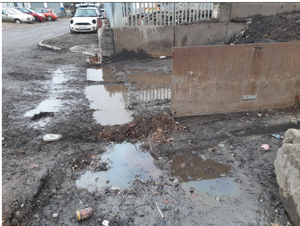
Photo 1 – pooling of water next to dewatering bay flowing onto unmade ground
