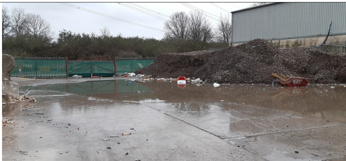
Photo 3 - Area of pooled water due to blocked drain at GD Environmental
