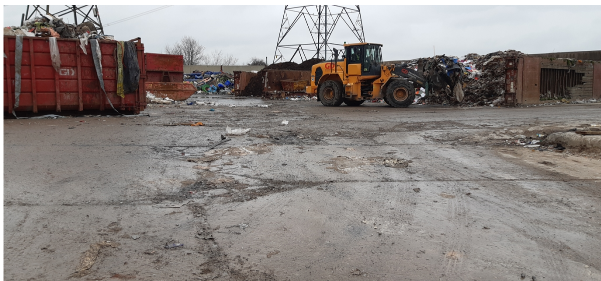
Photo 6 - Weakened areas of concrete flooring at GD Environmental
