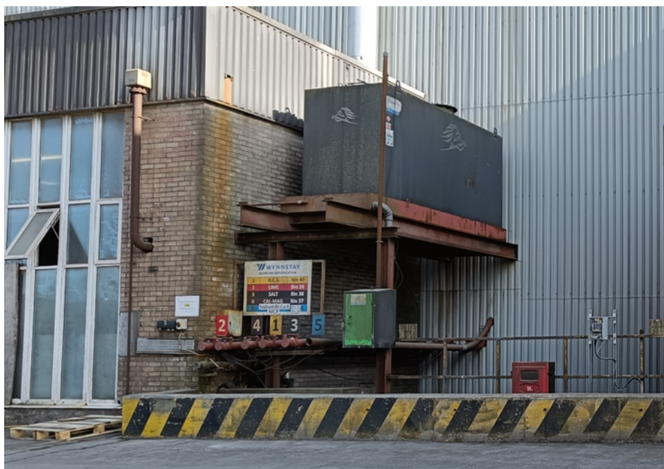
Kerosene storage tank in Bulk Loading Area
