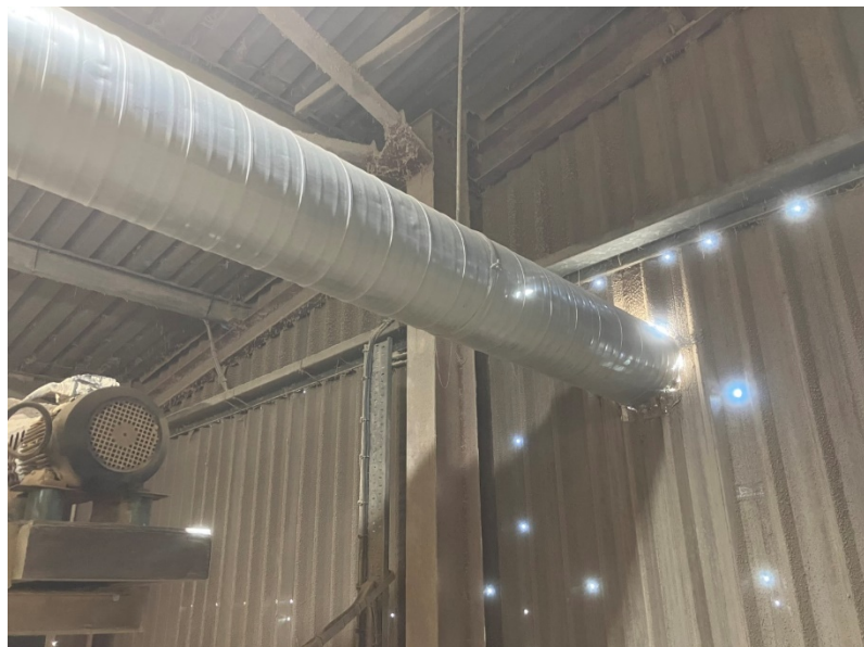
LEV22 Blend Bin extraction emission point to air
