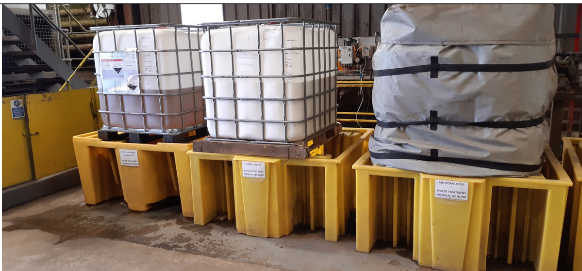
Photo 3 - Secondary containment bund for liquid storage
