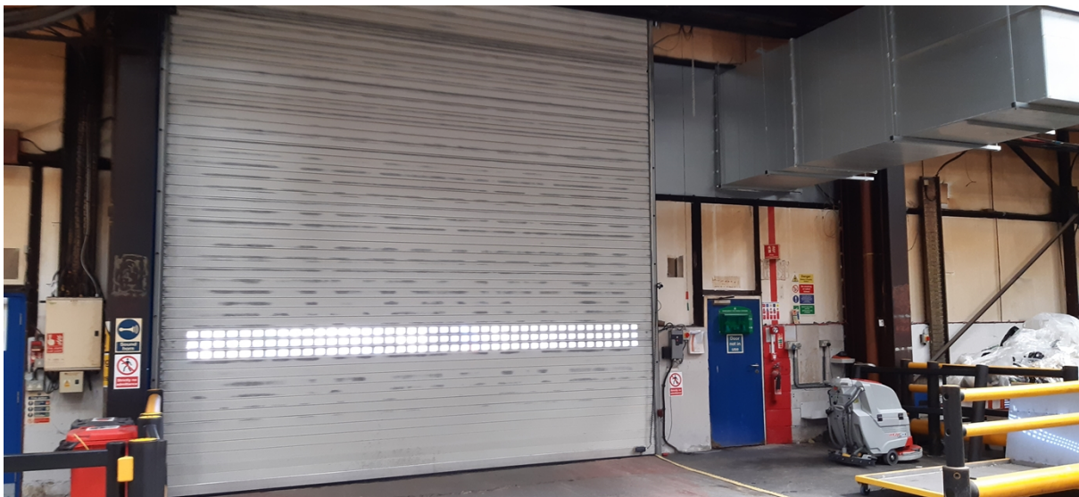
Photo 6 - Automatic roller shutter doors in operation during site visit
