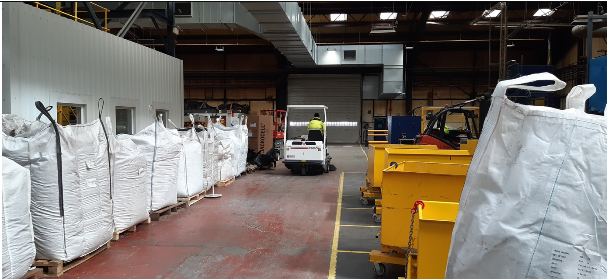
Photo 5 - Air Handling Unit (AHU) installed to mitigate excess noise emissions
