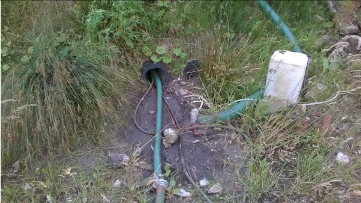
Photo 1 showing leachate risers. Note that run off is accumulating; in addition to a temporary separation bund the engineered ramp needs to be progressed.
