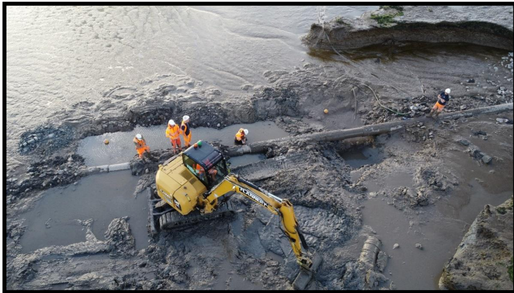
2) During the emergency slip-lining works (please note that the 9t excavator shown imposed a ground bearing pressure of approx. 39.8kN/m 2 ).
