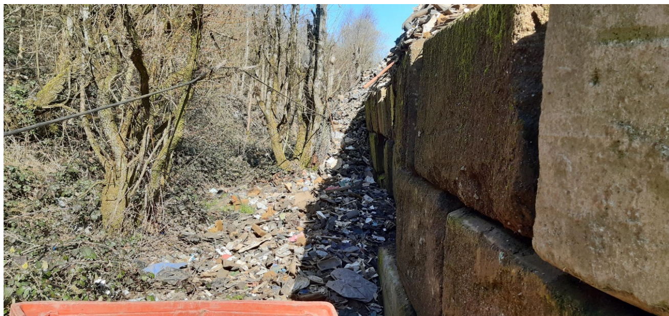
Photo 5 – waste has fallen from stockpile and damaged perimeter fencing
