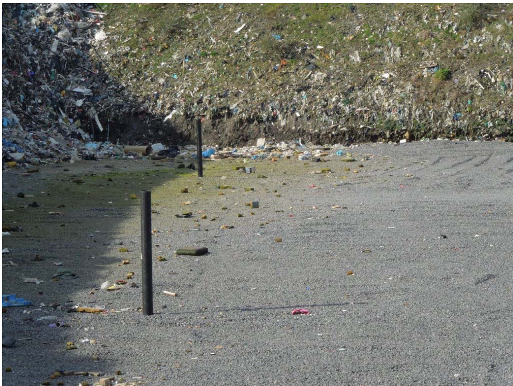
Gas Wells in Sub-Cell Base
