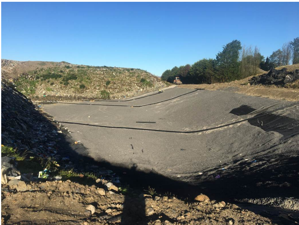
Leachate pipes in base
