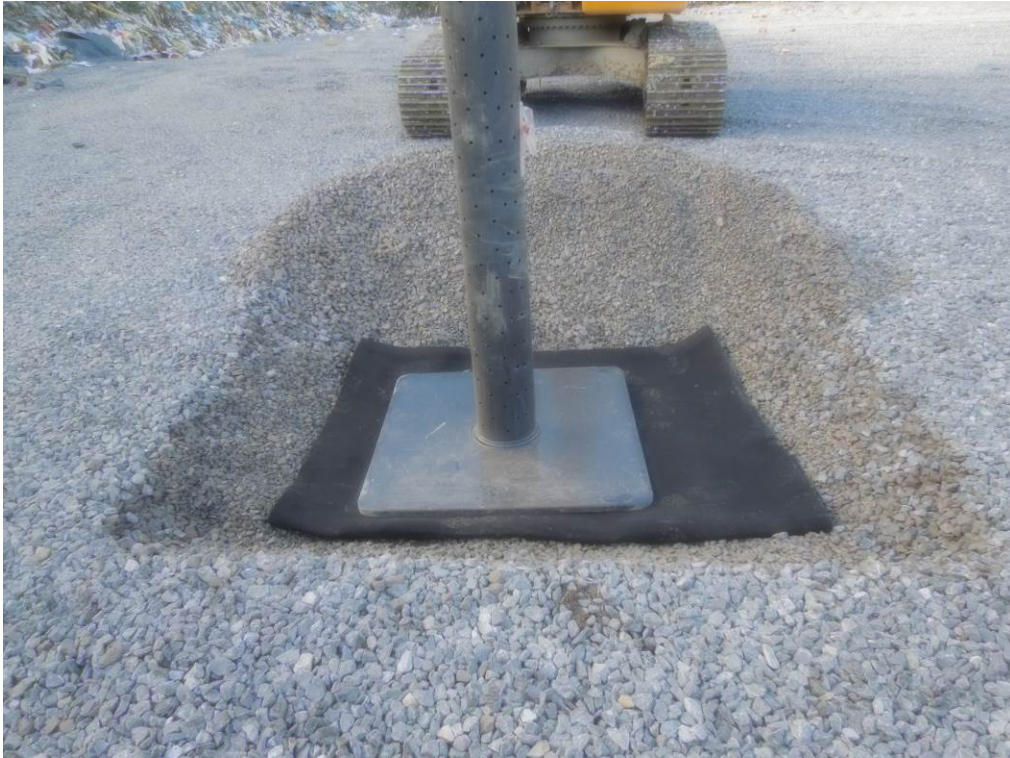
Gas Wells in Sub-Cell Base
