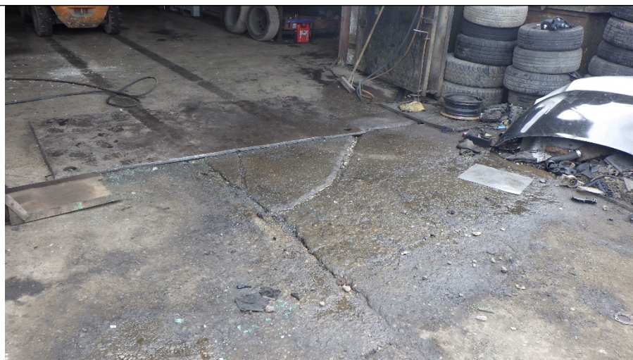
entrance to the depollution
