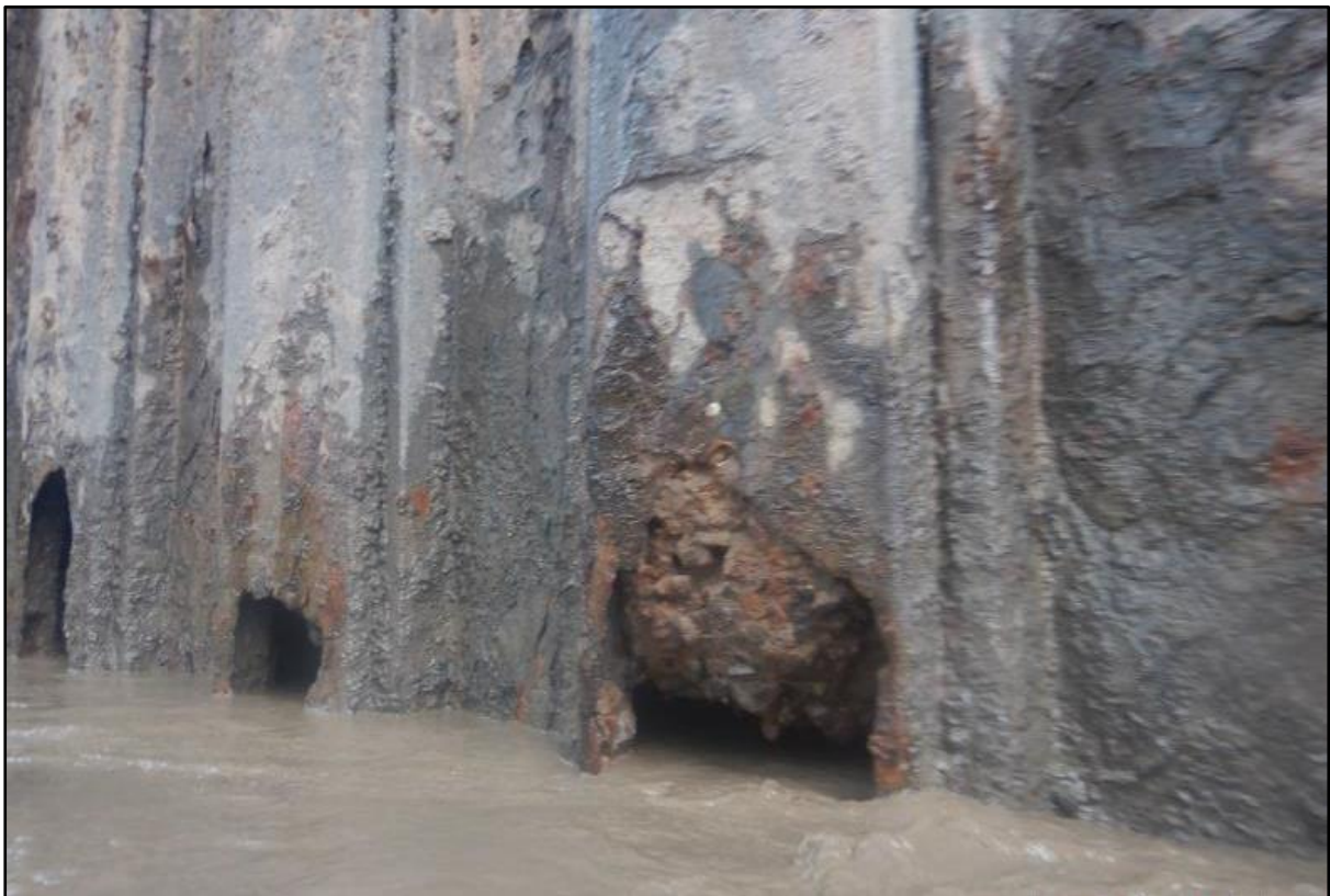
Figure 1.8 – Old Wye Bridge Pier 2, close up of corrosion to sheet piles
