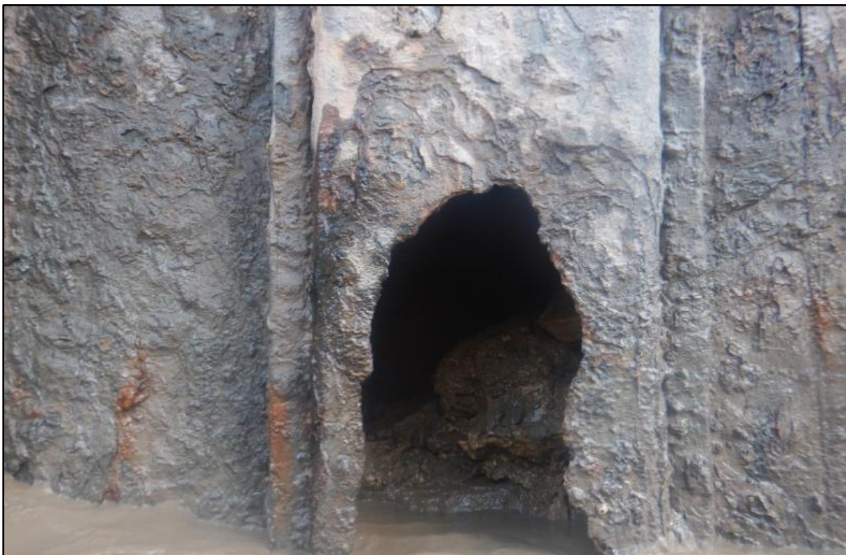
Figure 1.10 – Old Wye Bridge Pier 2, close up of corrosion to sheet piles
