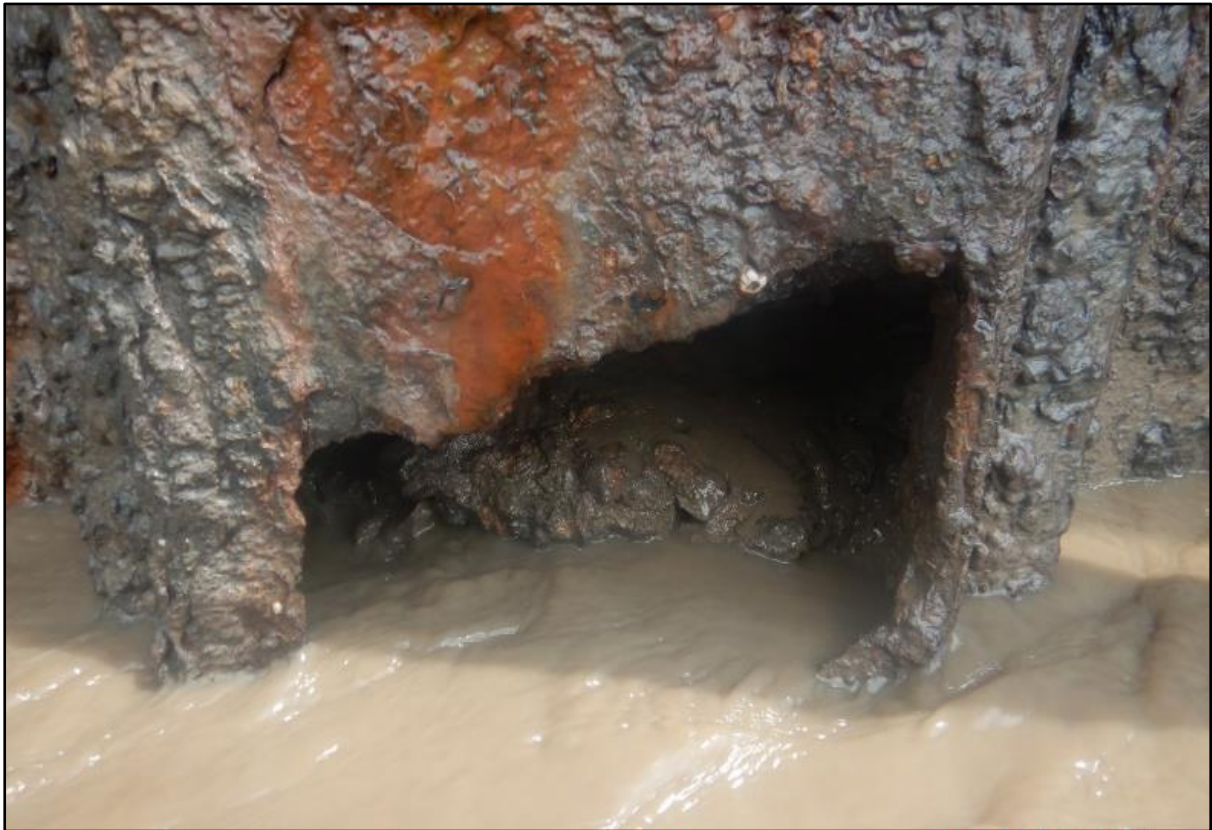
Figure 1.7 – Old Wye Bridge Pier 2, close up of corrosion to sheet piles
