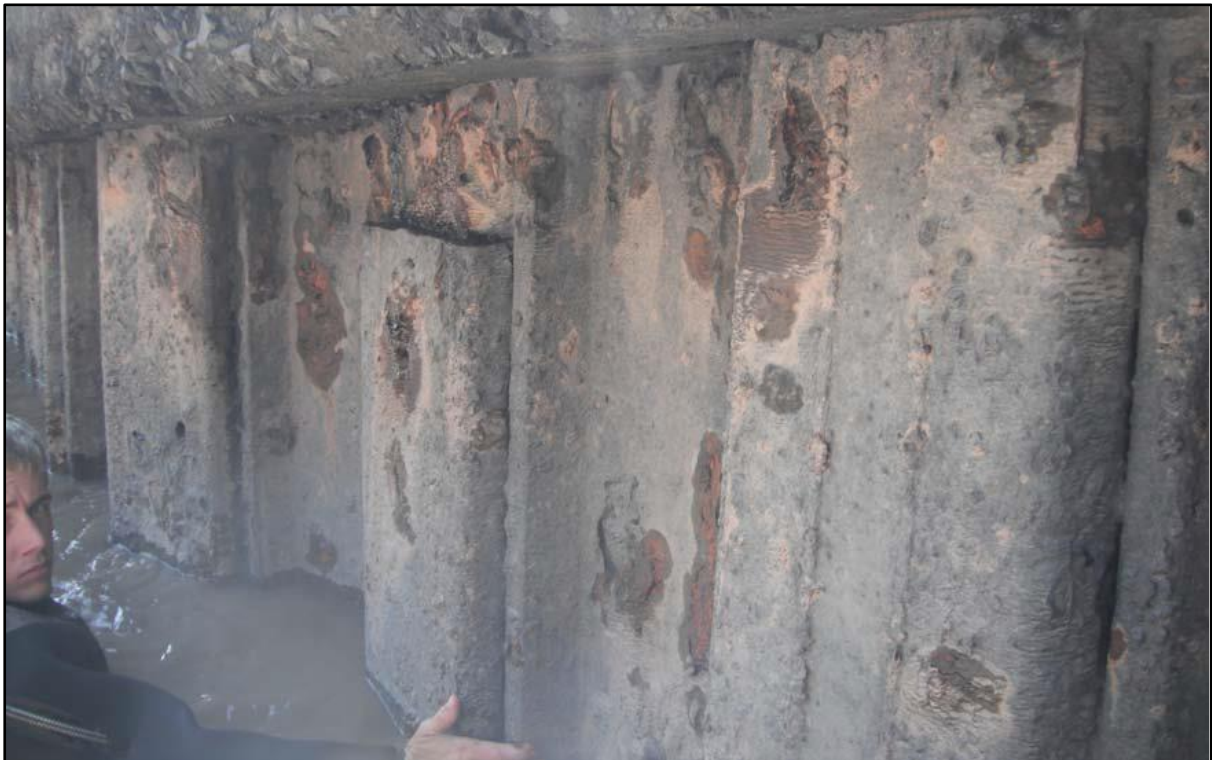
Figure 1.6 – Old Wye Bridge Pier 2, close up of corrosion to sheet piles, pier 2
