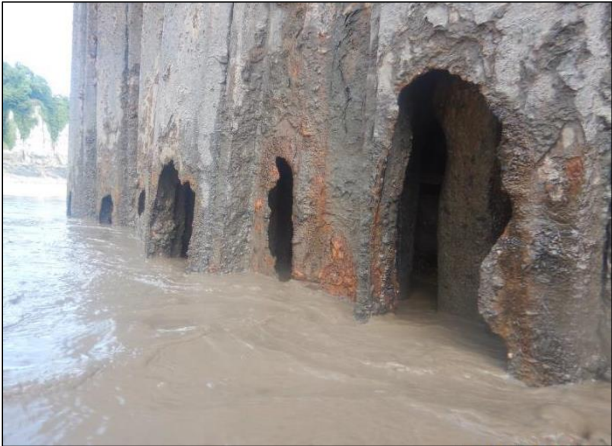
Figure 1.9 – Old Wye Bridge Pier 2, close up of corrosion to sheet piles
