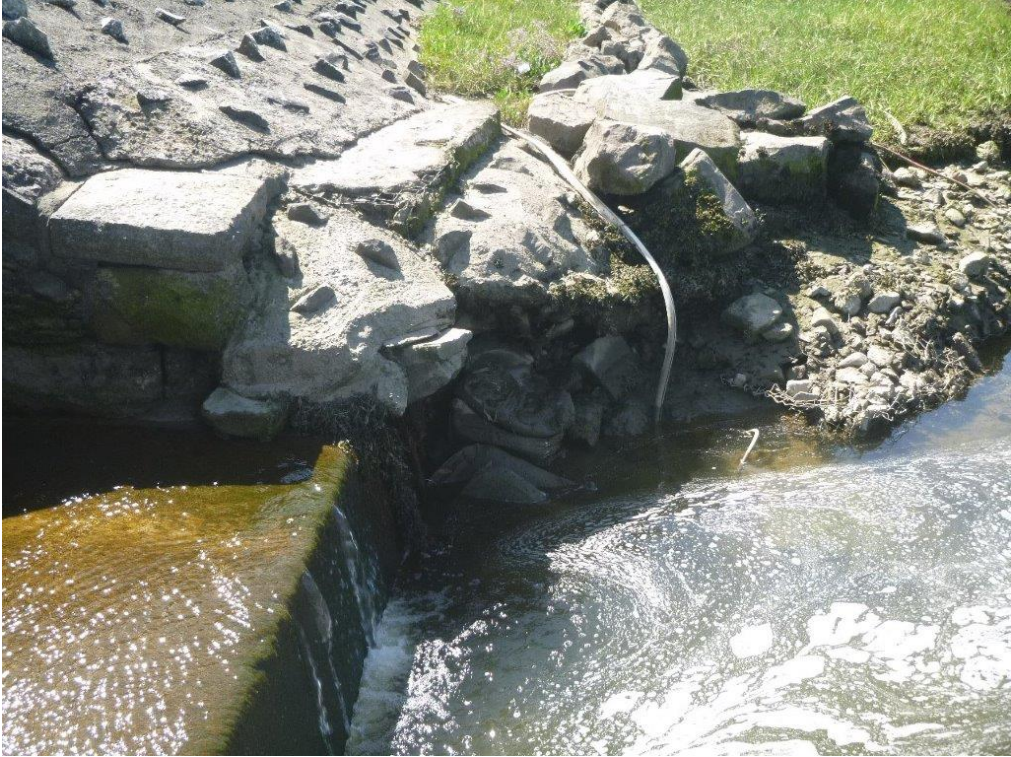
Photo 11 - Live significant defect (Taken 040822)
