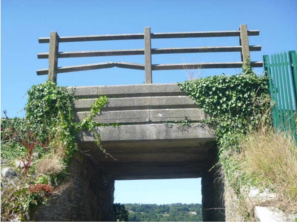
Photo 7 - Vegetation to downside elevation parapet 2sqm (Taken 040822)
