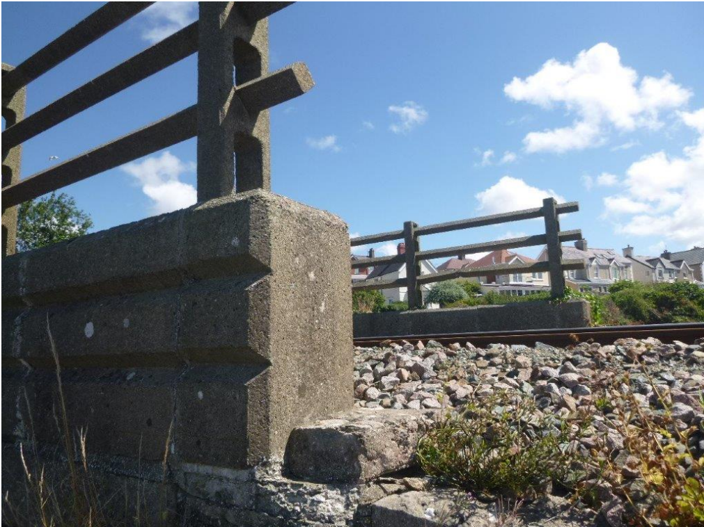
Photo 15 - Live significant defect (Taken 040822)
