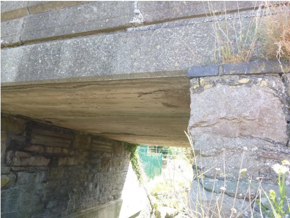
Photo 14 - Live significant defect (Taken 040822)
