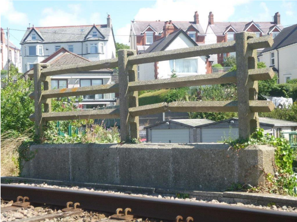
Photo 10 - Live significant defect (Taken 040822)
