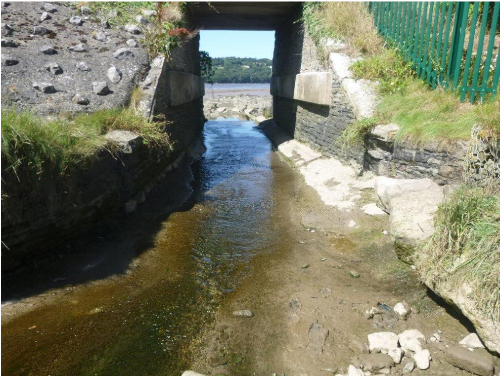
Photo 18 - Live significant defect (Taken 040822)
