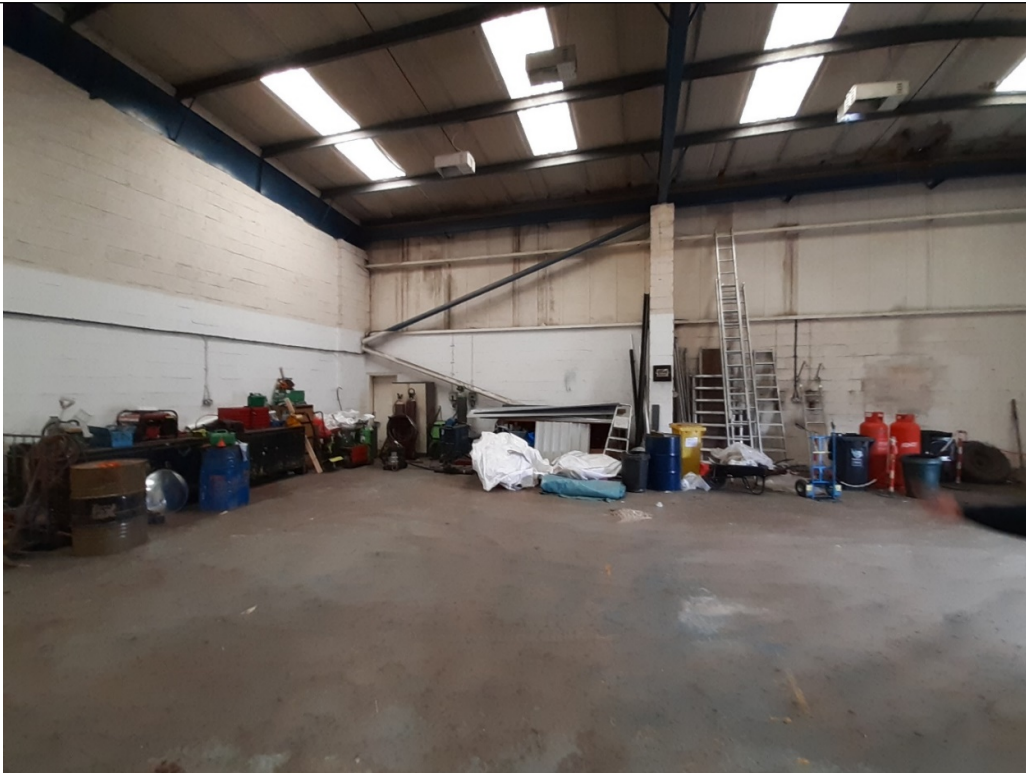
Photo 3 – inside unit 31. Flooring consists of hardstanding with no issues apparent infrastructure on site at time of inspection.
