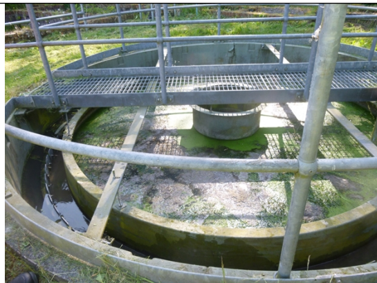
Humus tank in operation.
