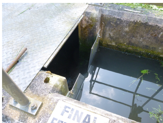
Final Effluent chamber, which was free from fungus and growth.
