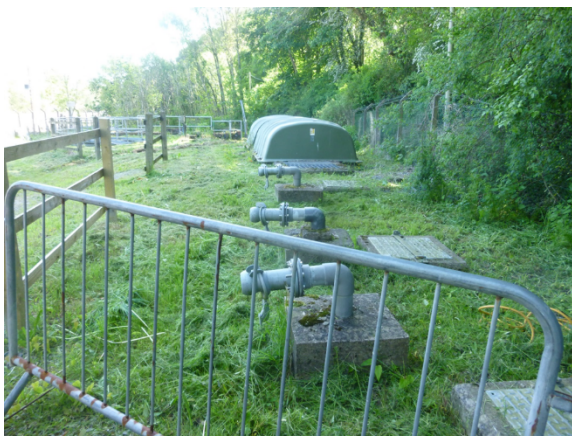
The sludge tanks are below ground, sludge is removed and taken to Kinmel bay for further processing
