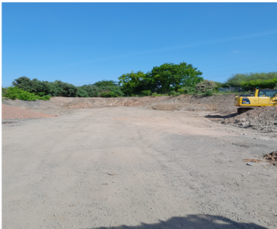
Photo 2 – Several piles of waste materials
