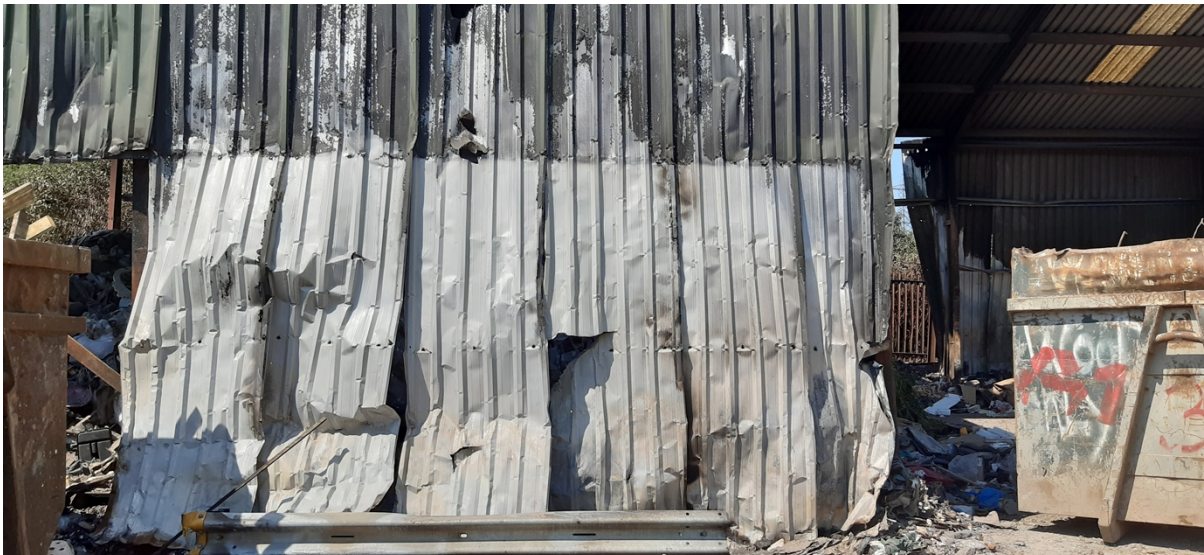
Photo 4 - Photo of fire incident taken by NRW Officer Greg GARDNER on 13/06/23
