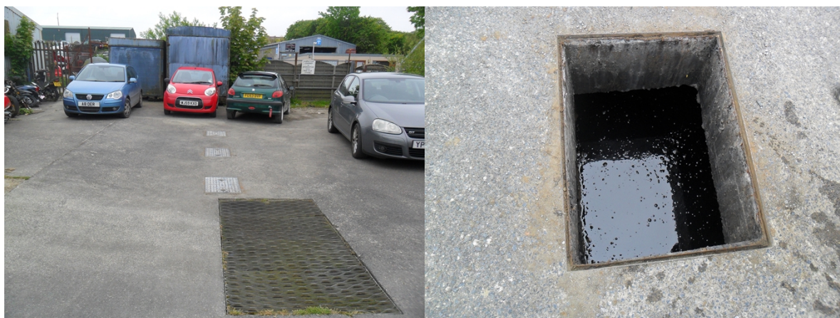
Photos showing interceptors rear of site office and the oil layer inside an interceptor
