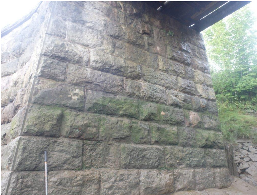
Photo 31: Low Mileage Abutment (02/08/22)
