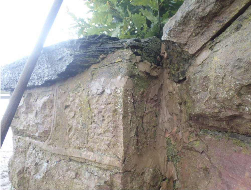
Photo 53: Newel stone shattered with spalled coping above, US LM Wing Wall (02/08/22)
