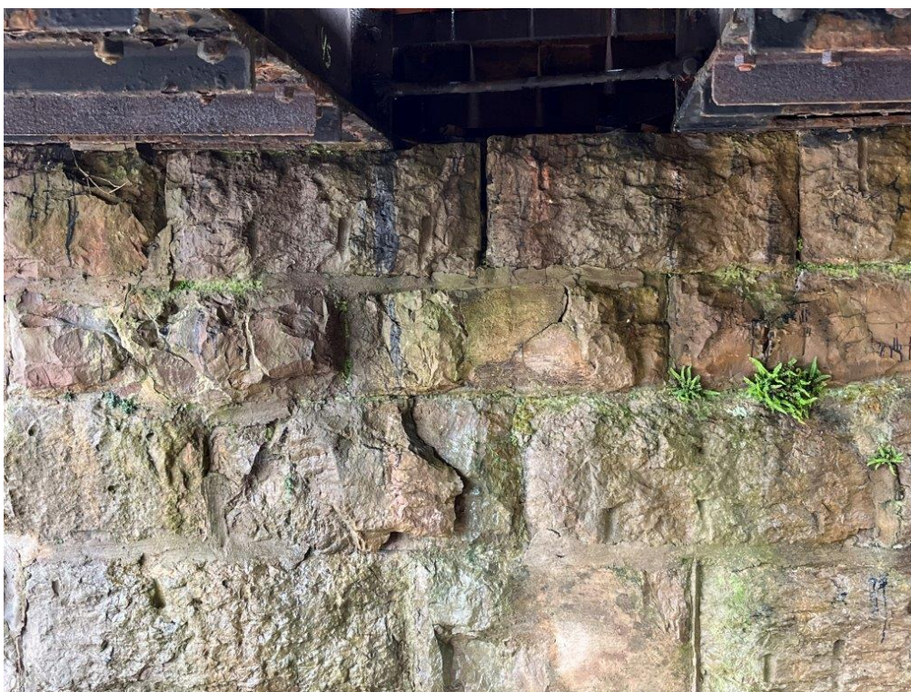
Photo 32: Area of split stones to LM Abutment (02/08/22)
