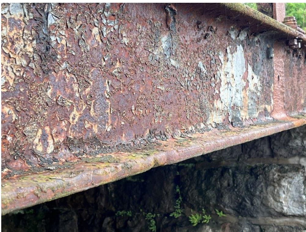
Photo 16: Area of notching to US Walkway Support Girder, HM 1/4 point (02/08/22)
