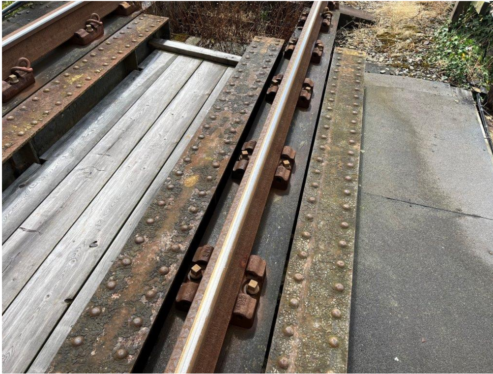
Photo 65: Missing clips prior to replacement (02/08/22)
