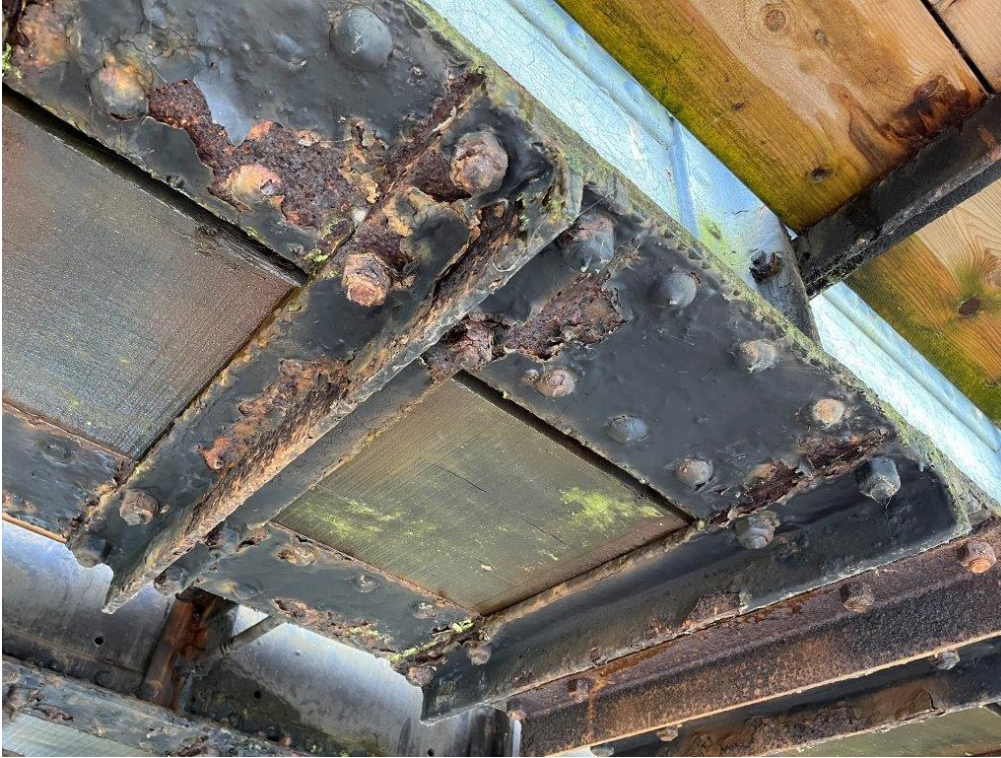
Photo 25: Further view of corrosion loss to US Main Girder (02/08/22)
