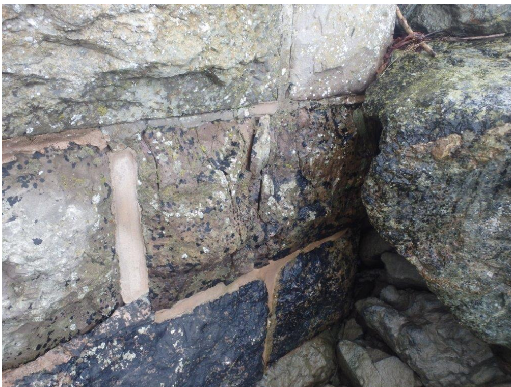
Photo 48: Shattered stone to Newel, US HM Wing Wall (02/08/22)
