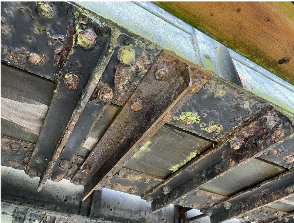
Photo 24: Typical corrosion loss to US Main Girder (02/08/22)
