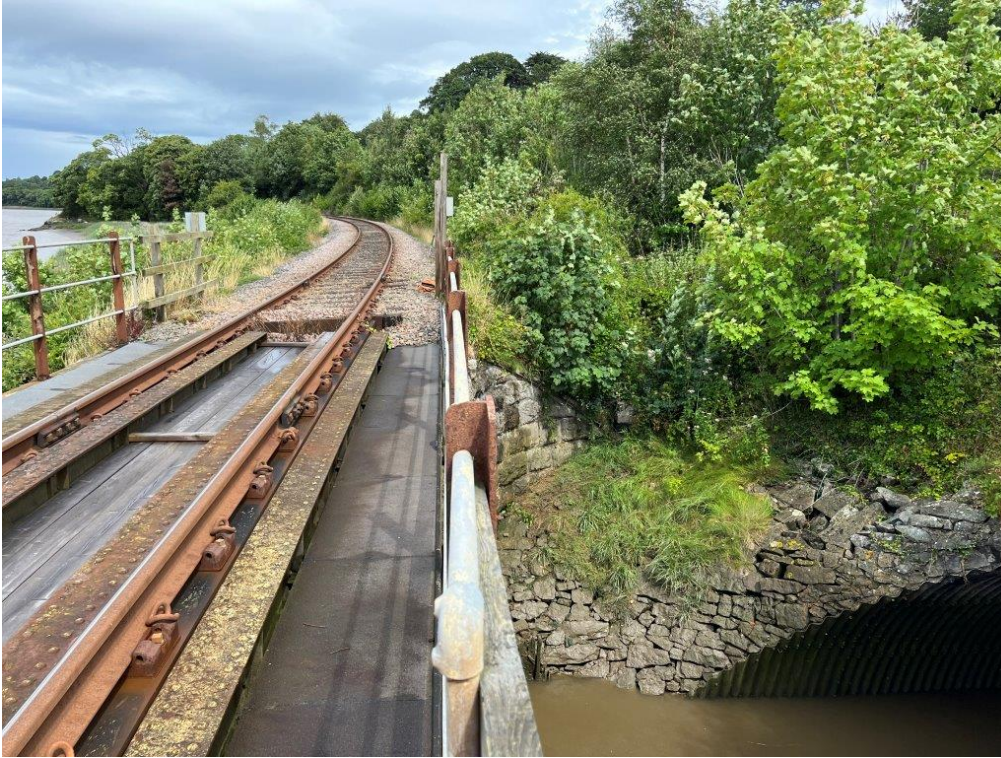
Photo 63: Downside Handrails appearing to bow (02/08/22)
