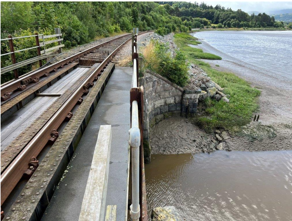
Photo 64: Poor profile to US Handrails (02/08/22)
