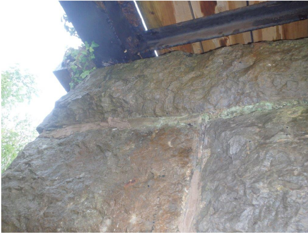
Photo 37: 1no stone to DS quoin, top course, set forward 10mm (02/08/22)
