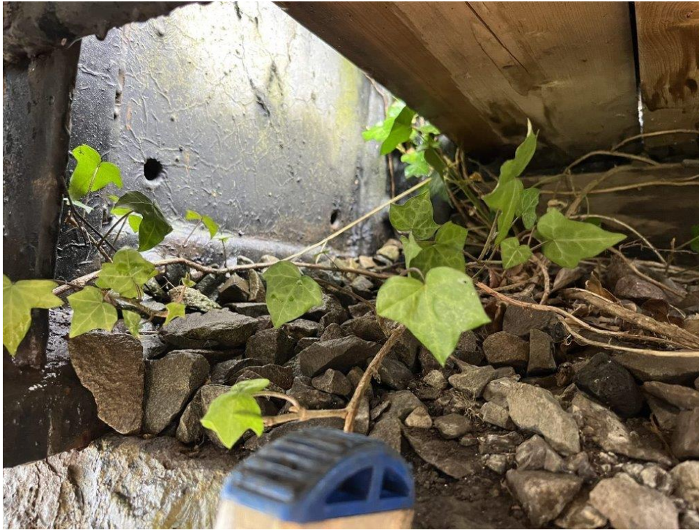
Photo 55: Typical view of ballast/debris to bearing shelf/Abutment (02/08/22)
