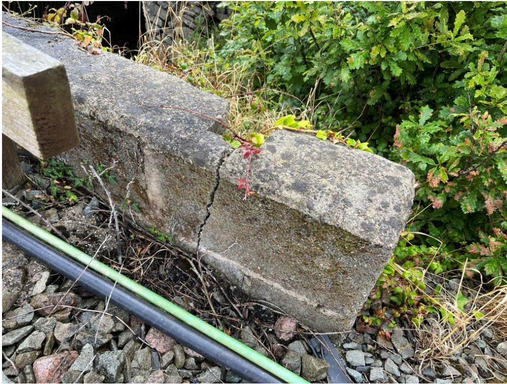
Photo 57: Typical fracture to Ballast Wall (02/08/22)
