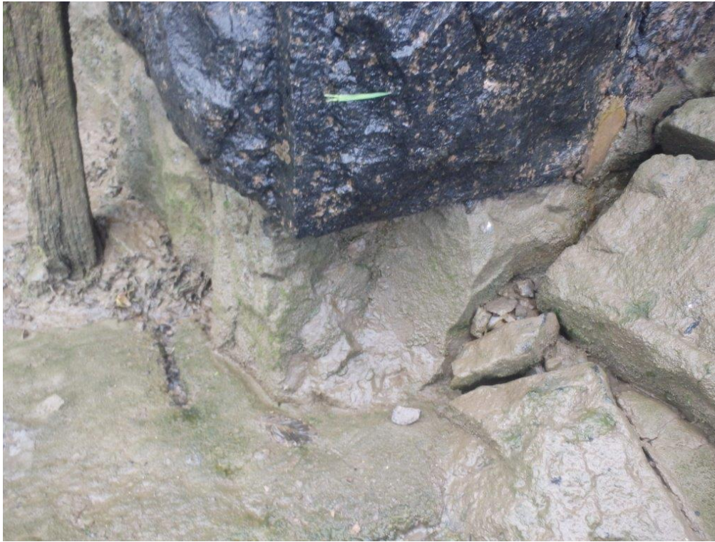
Photo 47: Newel quoin stone spalled to 150mm, US HM Wing Wall (02/08/22)
