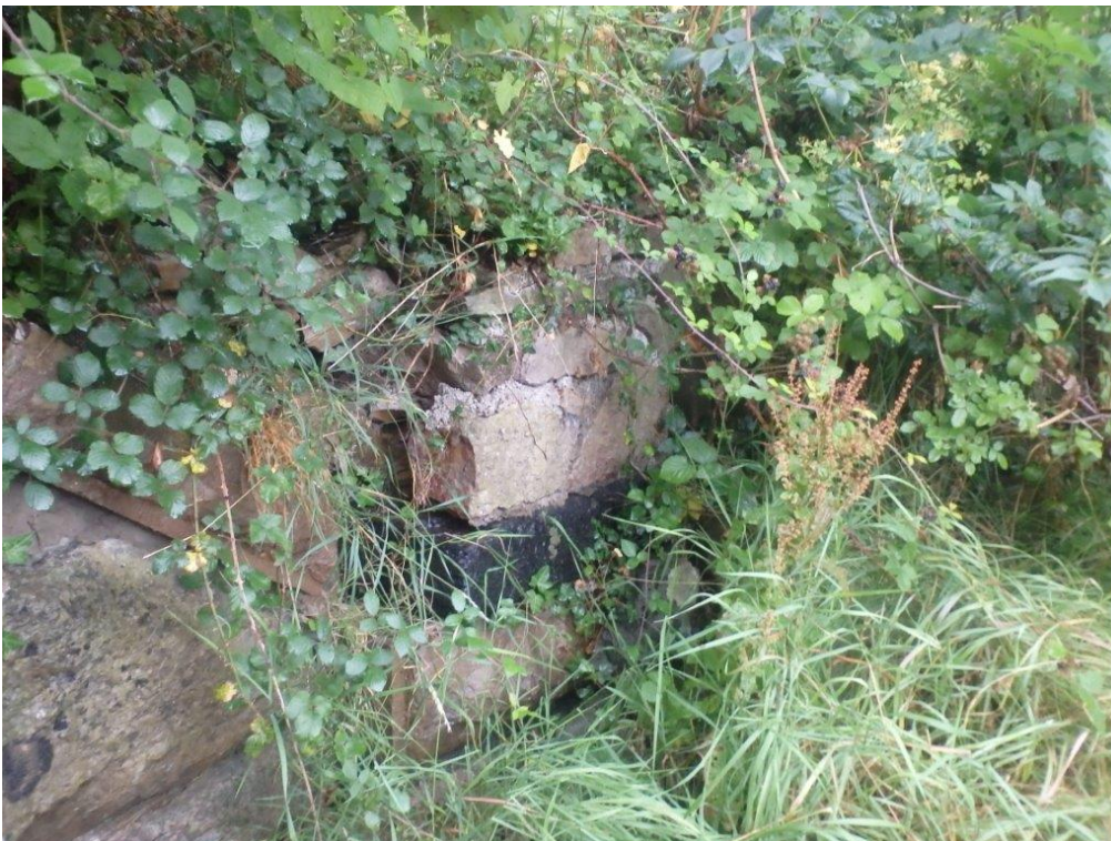
Photo 44: Displaced/missing to Newel and adjacent Retaining Wall (02/08/22)
