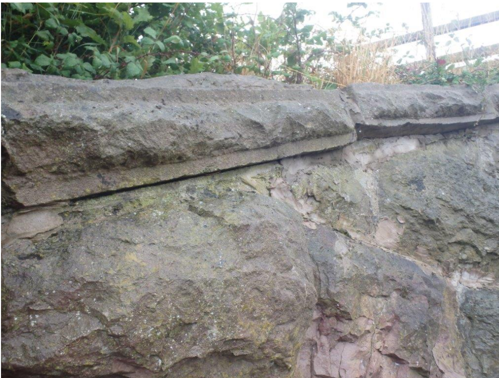
Photo 52: Bed joint fracture below copings, US LM Wing Wall (02/08/22)
