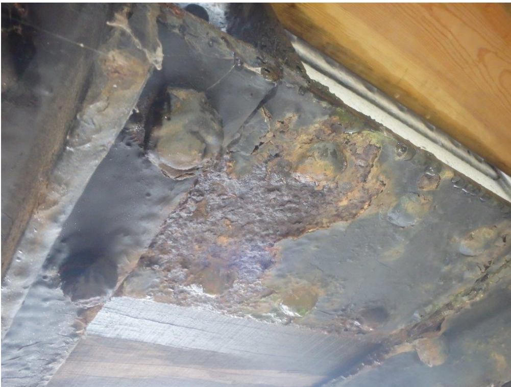
Photo 26: Increased corrosion loss to US Main Girder at connections (02/08/22)
