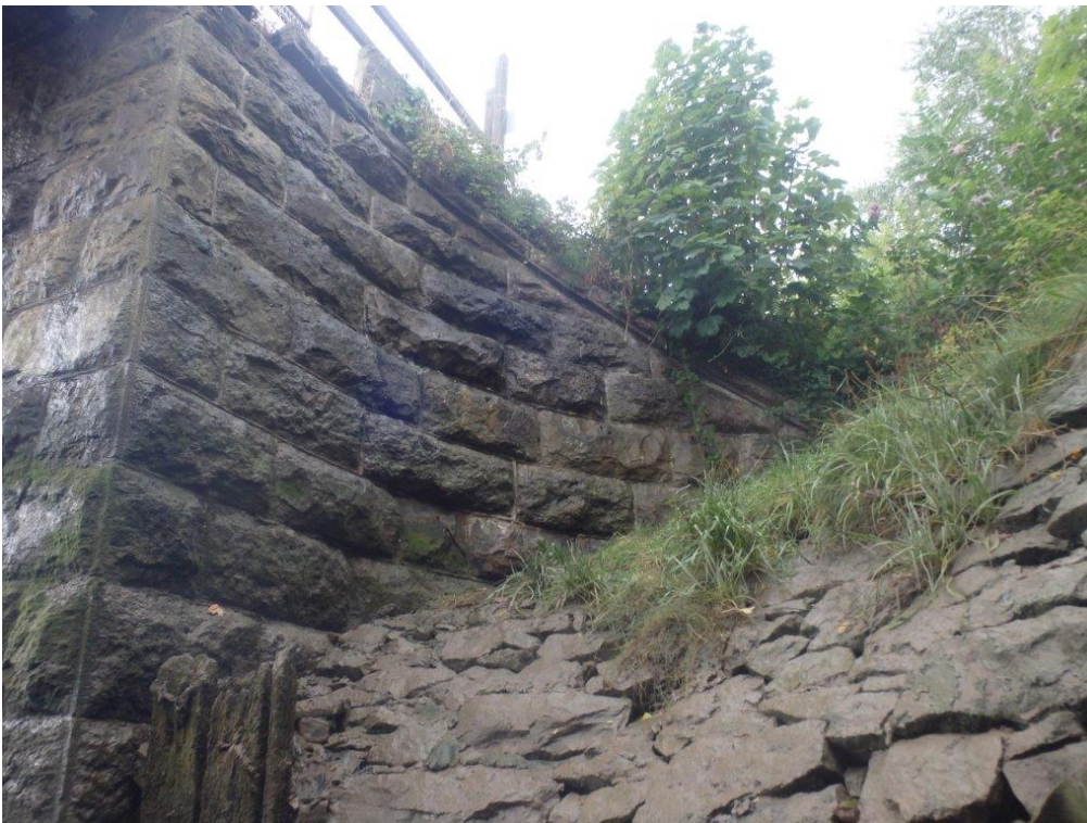
Photo 42: Downside Low Mileage Wing Wall (02/08/22)
