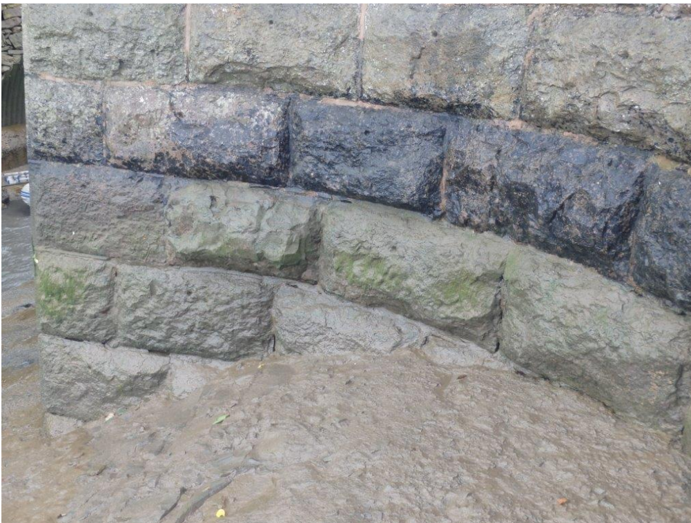
Photo 46: OJs to US HM Wing Wall (02/08/22)
