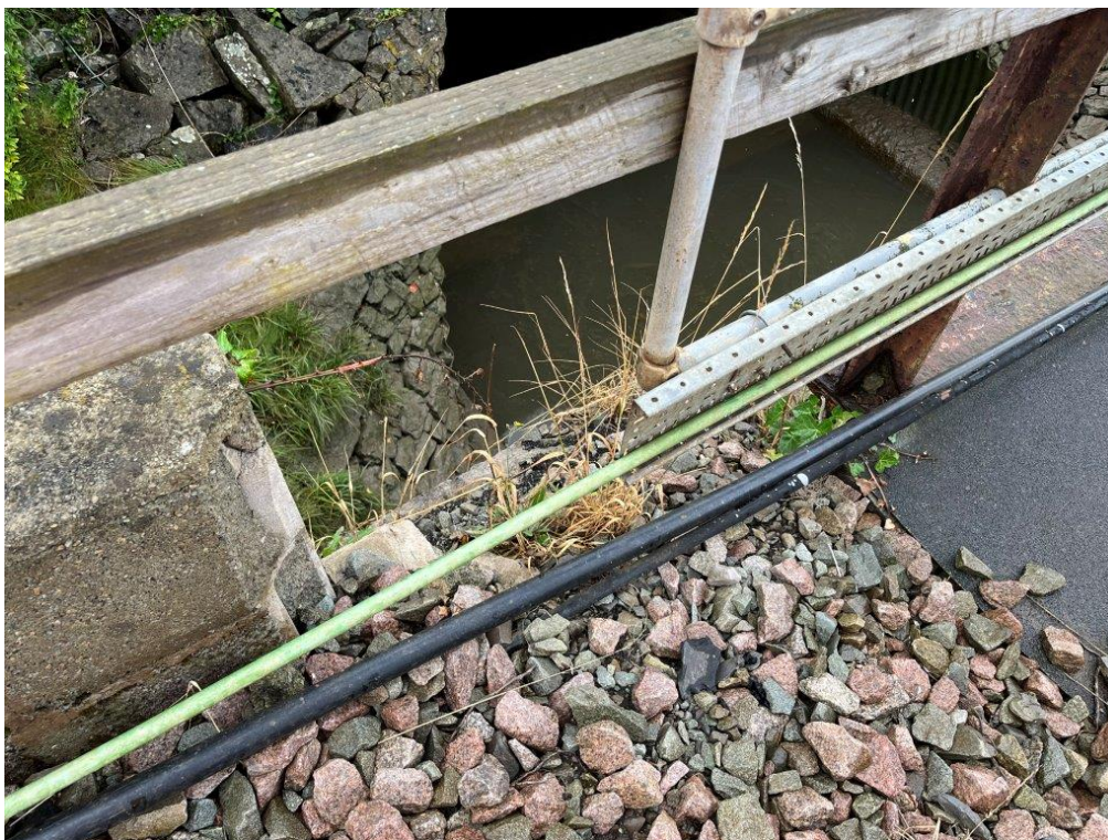
Photo 58: Section of DS LM Ballast Wall now missing (02/08/22)
