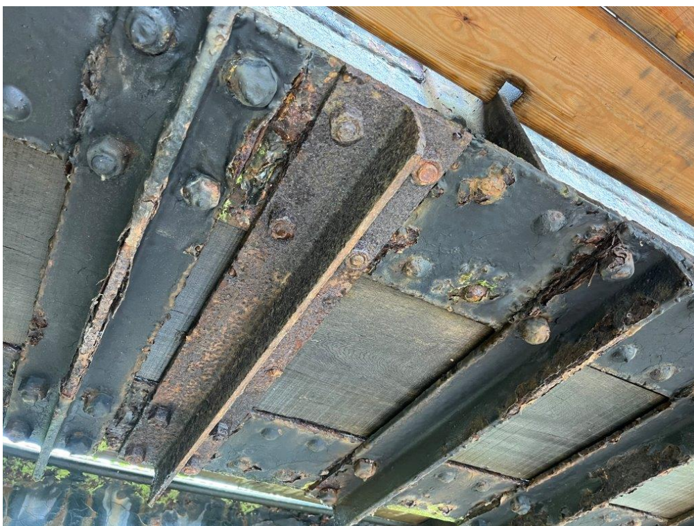
Photo 20: Typical view of condition of DS Main Girder, note corrosion loss at connections and lamination (02/08/22)
