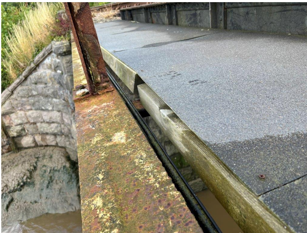
Photo 30: Displacement to US Walkway (02/08/22)
