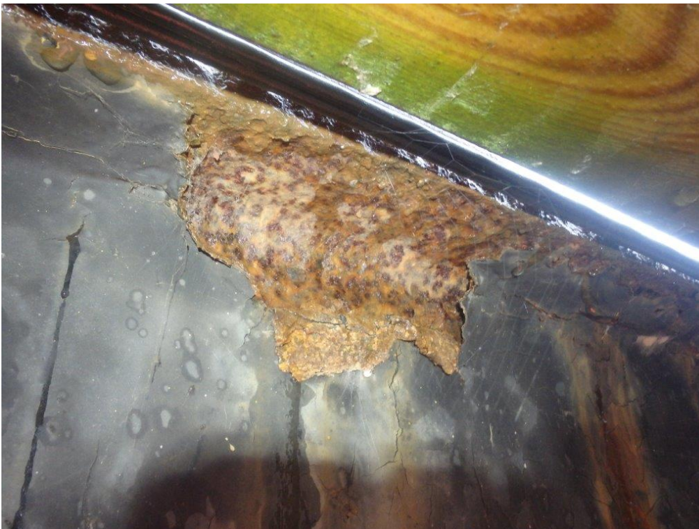
Photo 14: Odd example of corrosion loss to US Walkway Support Girder (02/08/22)
