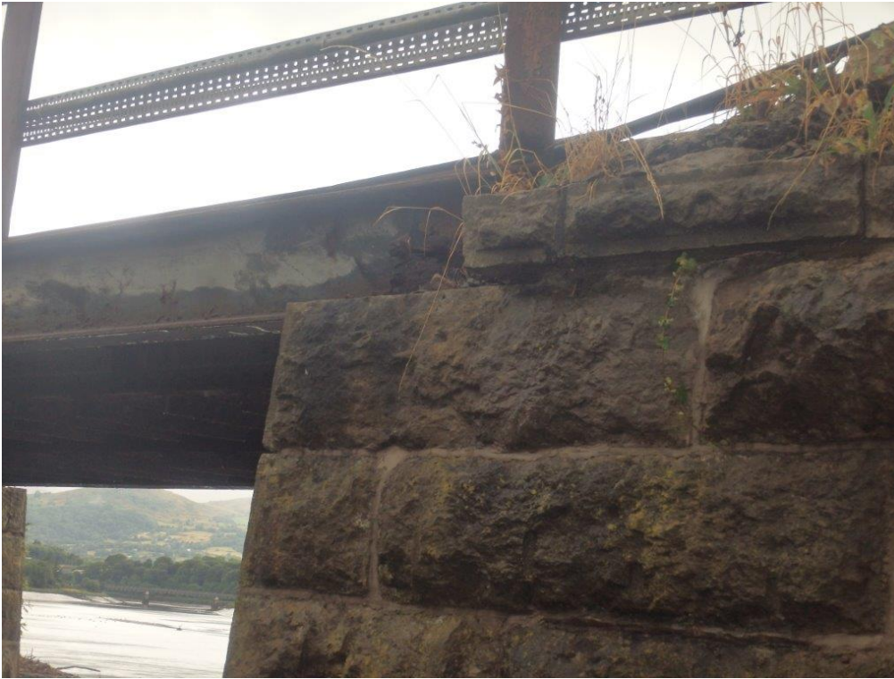
Photo 43: Missing top coping stone, DS LM Wing Wall (02/08/22)
