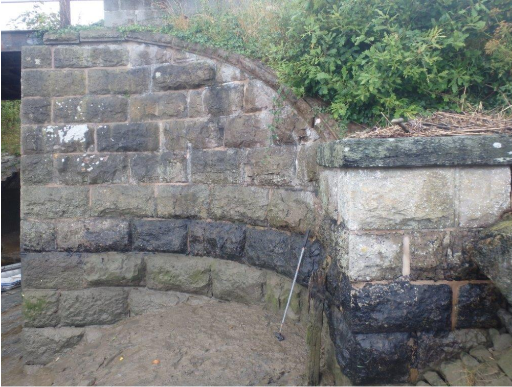
Photo 45: Upside High Mileage Wing Wall (02/08/22)
