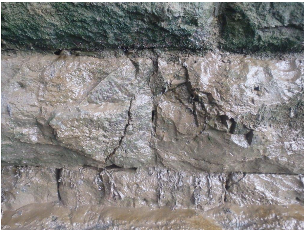
Photo 38: 1no split stone to HM Abutment with stone adjacent split to its corner (02/08/22)
