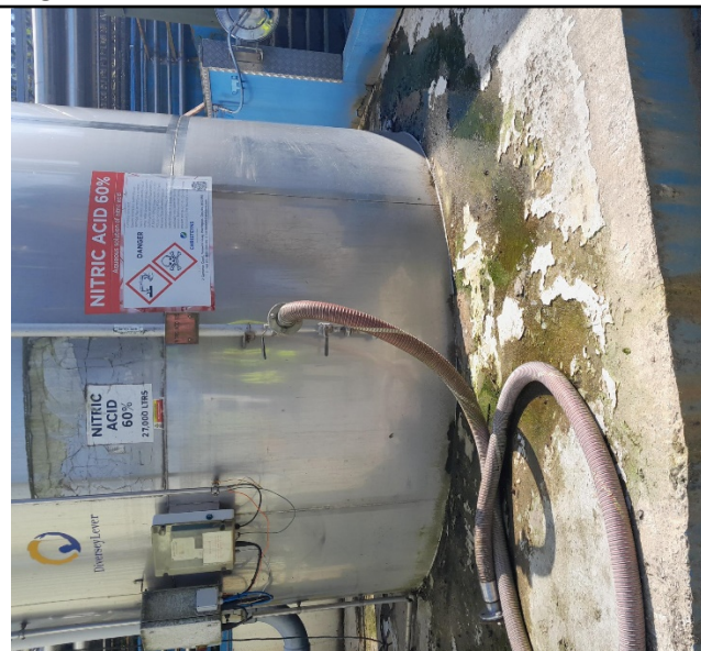
Pic 6. Nitric acid tank. Clarification is sought from site regarding the design specification of this unit as it reportedly has an integrated secondary bund. ACTION - Site to send unit spec to confirm ASAP. Signs of concrete corrosion can be seen. A hose is left to coil on the floor where it could degrade in any residual acid left there.
