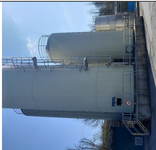
Pic 3 Existing tanks showing single skin, no secondary containment. Site relies upon perimeter tertiary containment to collect spillages which are directed to the on-site Effluent treatment plant.
