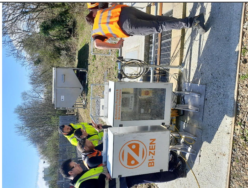
Pic 12. The sub surface holding tank in position upstream of the ETP. (installed at the same time the ETP was constructed). Site was undergoing trials of new probes in the effluent flow which show pH, turbidity, and flow rate into the ETP.
