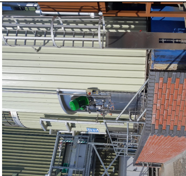
Pic 7. Above, this tank had a half bund wall for protection against traffic but no secondary containment.
