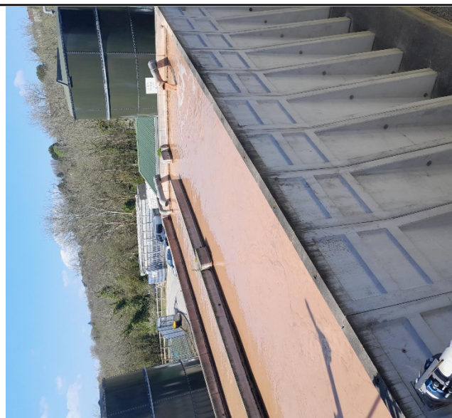
Pic 10. The ETP aeration tank 'lanes' made from pre-stressed concrete panels.
