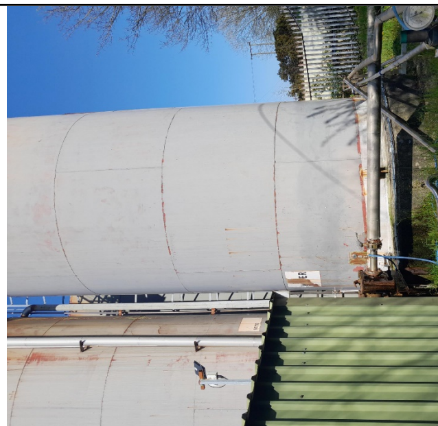
Pic 4. Single skinned tanks without secondary containment. The tank is showing signs of rust and needs to be placed on a scheduled maintenance regime.
