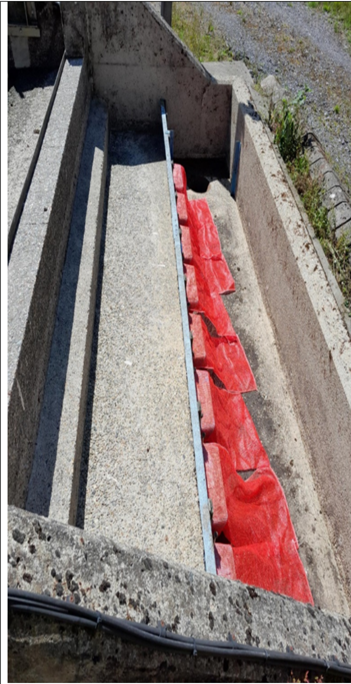
photo 2 : overflow weir to Storm with COPA sacs for extra screening.
