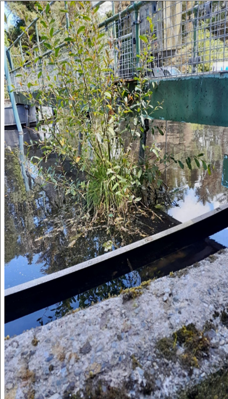
Photo 5: Final effluent tank
