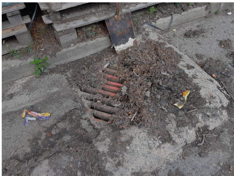
Second drain partially covered with street cleaning residues
