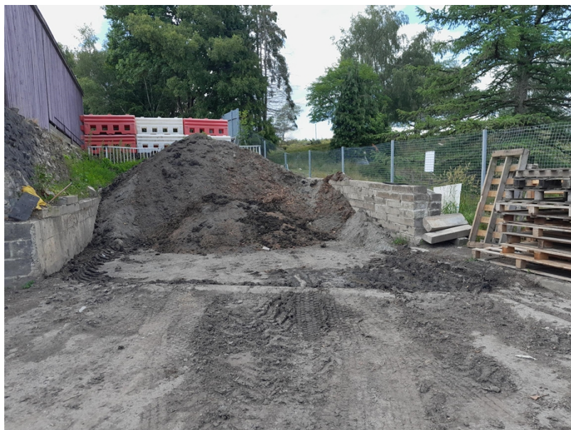
Dewatering bay with drain completely covered with street cleaning residues
