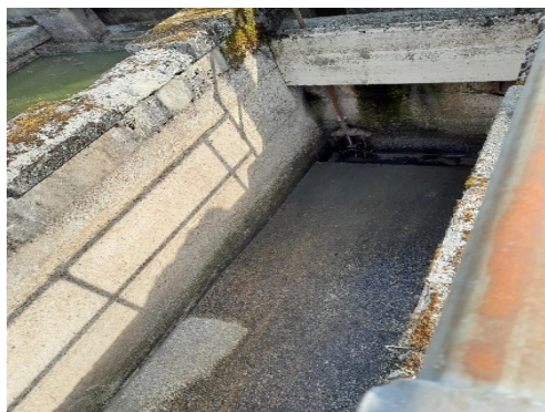
Image 3 – Storm tank, clean and empty.
