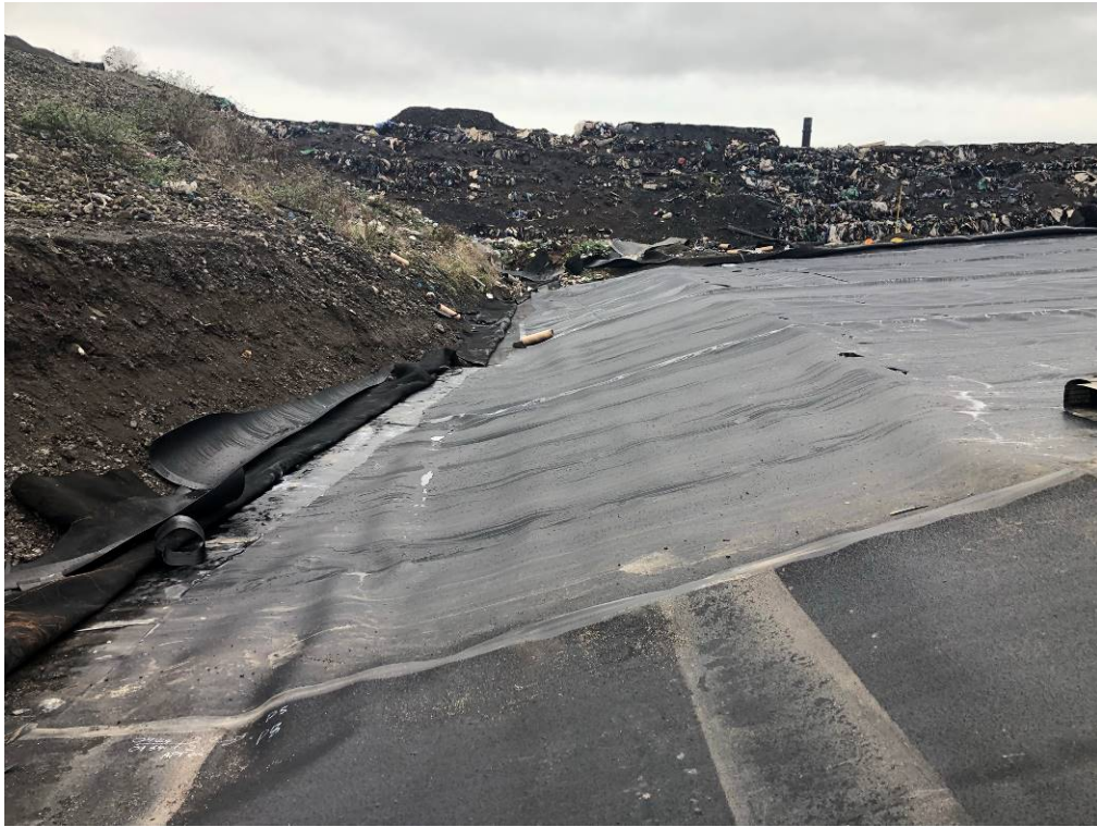
Toe connection with Biocells A & B
