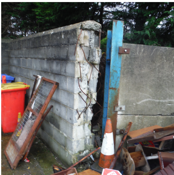
2. Gap in wall that needs to be filled in to prevent potential escape of fire water into the adjacent Afon Dulas.
