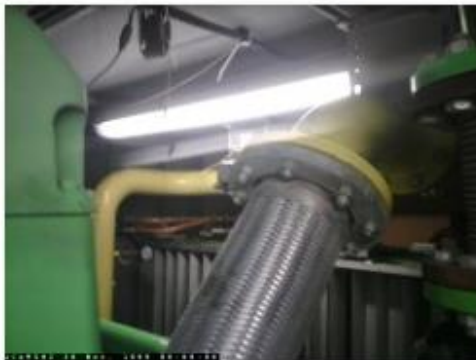
P58 CHP unit gas pipework
