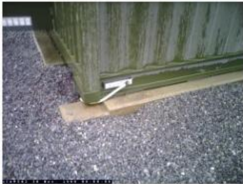
P55 CHP unit earthing
