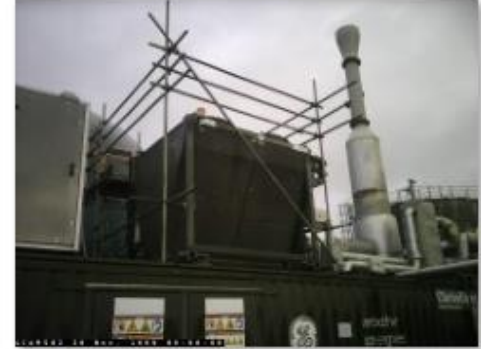
P54 CHP unit heat exchanger and exhaust stack
