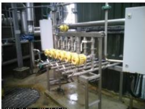
P28 isolated but not removed gas mixing system
