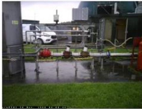
P47 biogas flare unit
