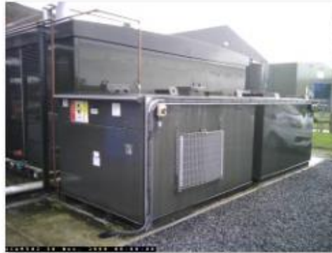
P8 CHP lube oil tanks
