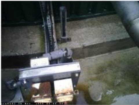
P34 corroded electrical switches adjacent to condensate trap
