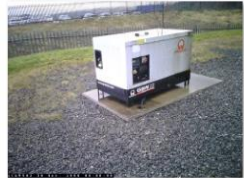
P3 emergency generator
