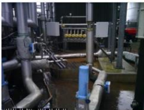
P26 congested plant area
