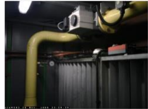
P57 CHP unit gas pipework
