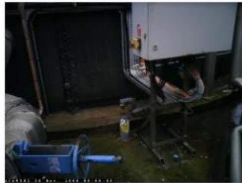
P23 condensate trap adjacent to electrical panel
