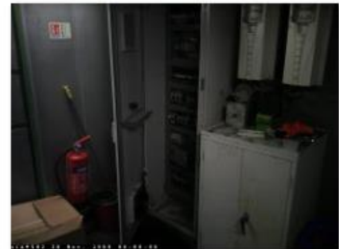
P60 CHP unit open control cabinet and fire extinguisher
