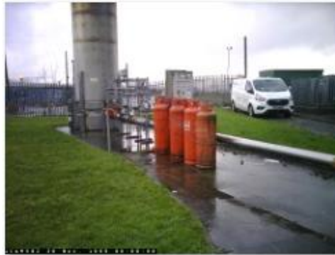
P2 propane cylinders at flare unit
