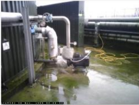
P37 process area and pumps
