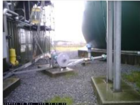
P41 bioqas storage membrane
