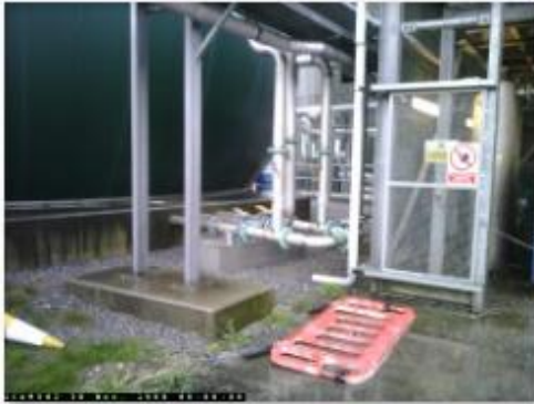
P43 biogas storage membrane
