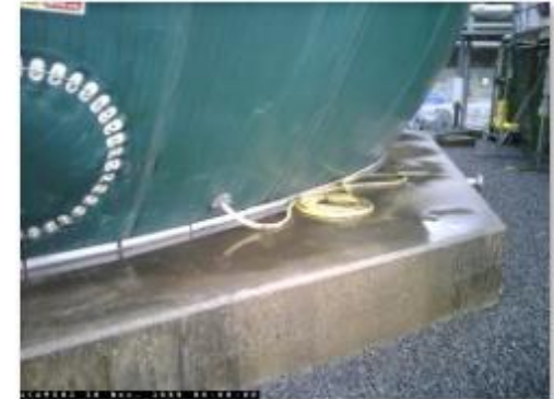
P42 bioqas storage membrane
