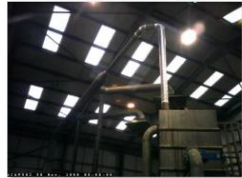
P15 odour control extract ductwork
