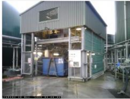
P14 separator room
