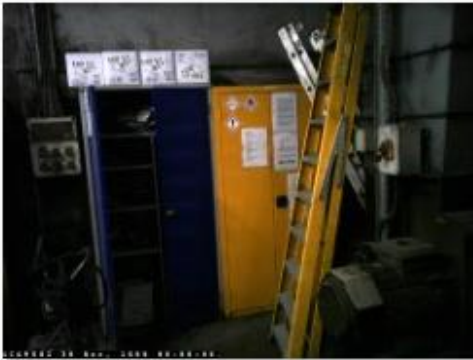
P7 flammables cabinet
