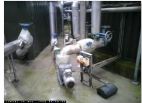
P36 process area and pumps
