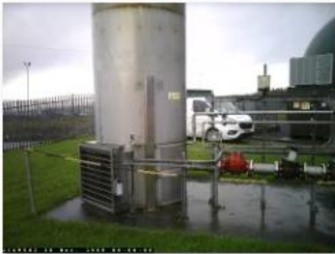
P46 biogas flare unit
