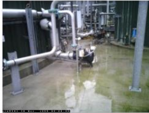
P32 process area and pumps
