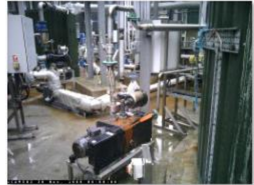
P33 process area and pumps
