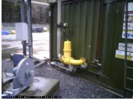
P52 CHP unit gas AIV
