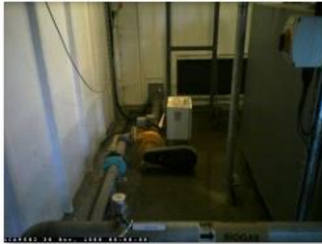
P49 biogas boiler unit
