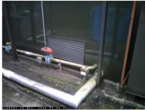
P50 biogas boiler unit
