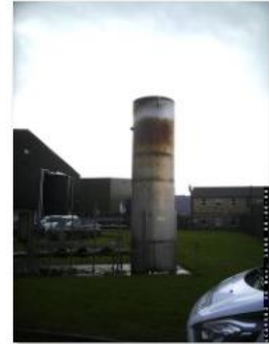
P45 biogas flare unit
