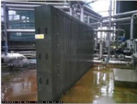
P31 heat exchanger
