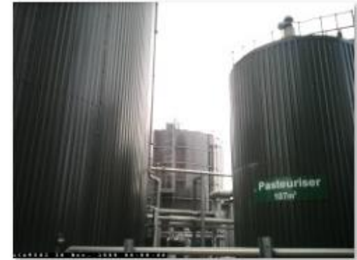
P39 digestate storage tank
