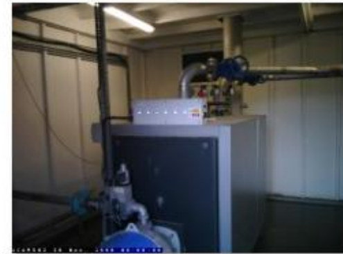
P48 biogas boiler unit
