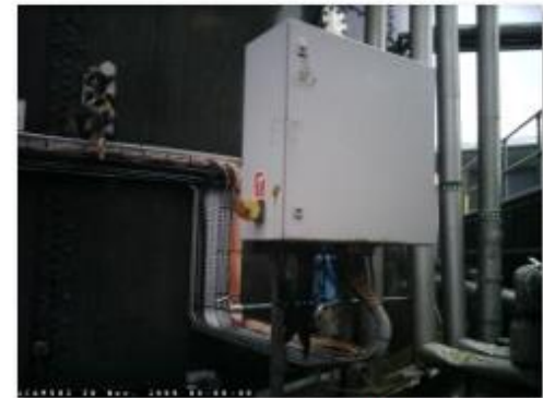
P24 electrical panel and plant e-stop
