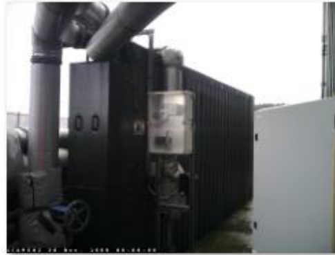
P38 heat exchanger
