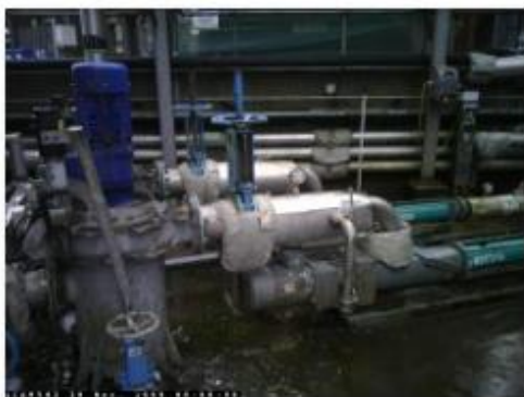
P25 feed pumps in congested area
