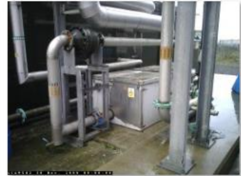
P51 CHP unit gas compressor
