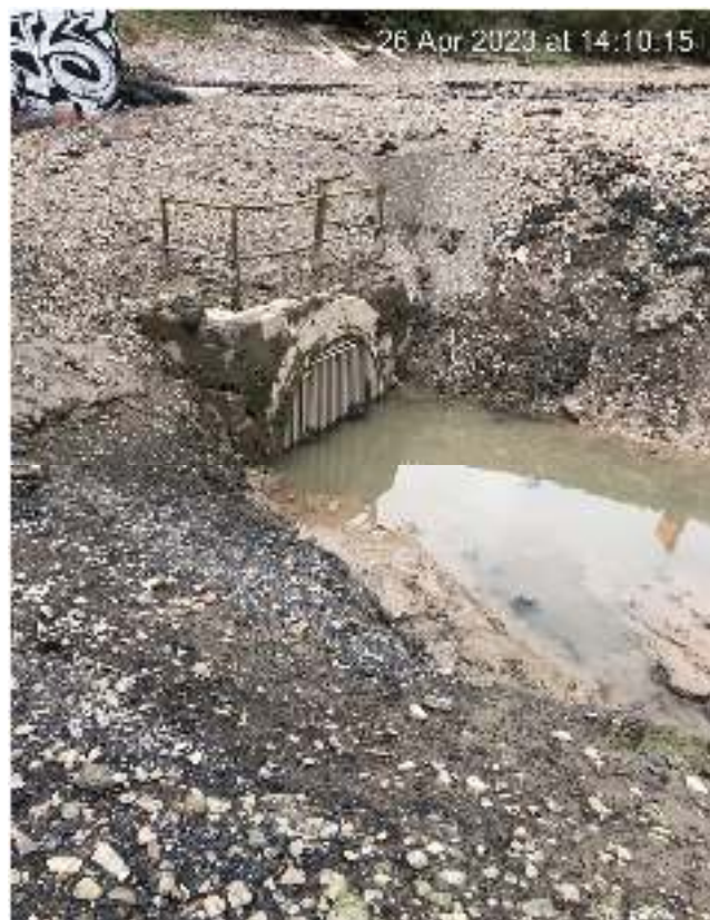
Figure 6 – area holding water.
