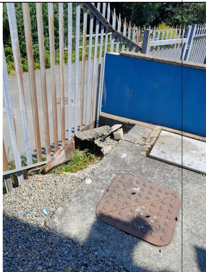
Fig 6 above. Shows the same drain in the road outside the fence with First Milk's overflow drain in the near ground. The overflow connected both drains. Concrete work has since blocked off the route from 7th June.
