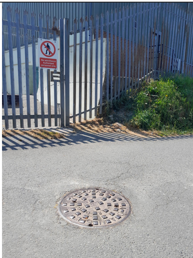
Fig 5 above. The same drain pictured outside the First Milk permitted fence line taken at the NRW inspection on 13 th June 2023.
