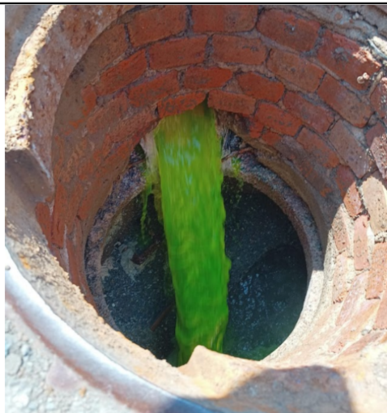
Fig 4 Taken by Dwr Cymru shows the same drain during dye tracing on 7th June by Dwr Cymru in the presence of First Milk staff. This confirmed the existence of the overflow pipe which allowed untreated effluent to overflow from the First Milk site into the Dwr Cymru
