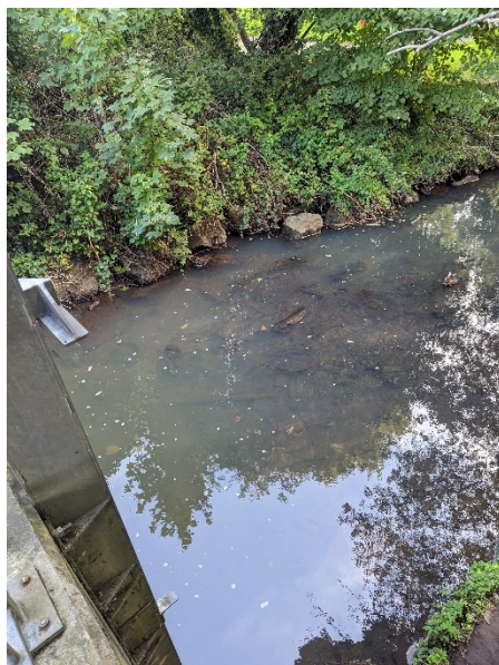
Figure 6. Grey, cloudy water exiting the culvert into Porset Brook.
