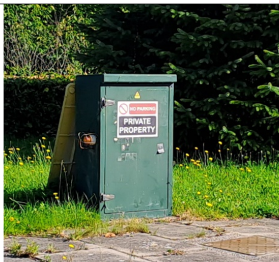
Figure 8. Secured control panel with warning light present but not on.
