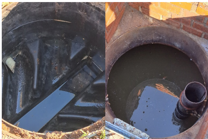
Figure 6 and 7. Chamber 1 and Chamber 2 free of solids and ragging.
