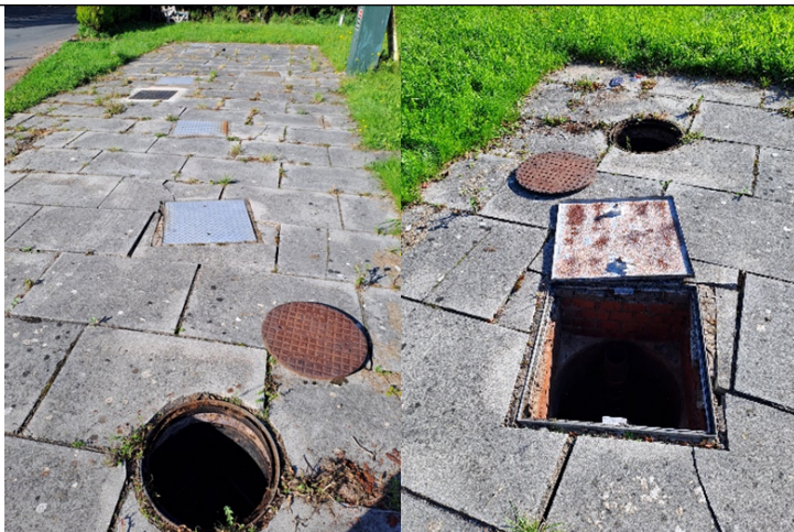
Figure 4 and 5. Location of PTP inspection chambers and chambers opened (inlet chamber 1 and secondary chamber 2).
