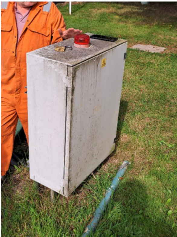
Figure 5. Control panel with warning light present but not alight.
