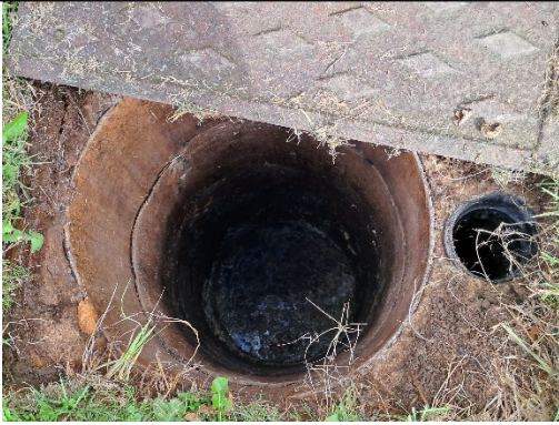
Figure 2. Primary receiving chamber.
