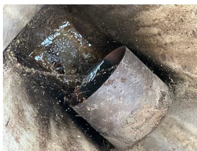
Sample Point Chamber (Photo 6)
